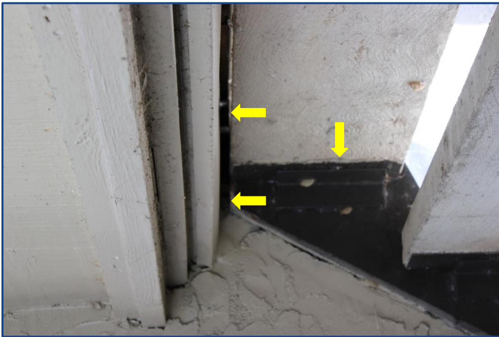
Photograph No. 18: Close-up view of the damages in Photograph No. 17.
