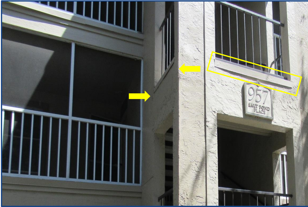
Photograph No. 13: Cracks in the stucco wall finish and corrosion and damage to the metal flashing at the edge of the stairway landing slab at the south stairway.
