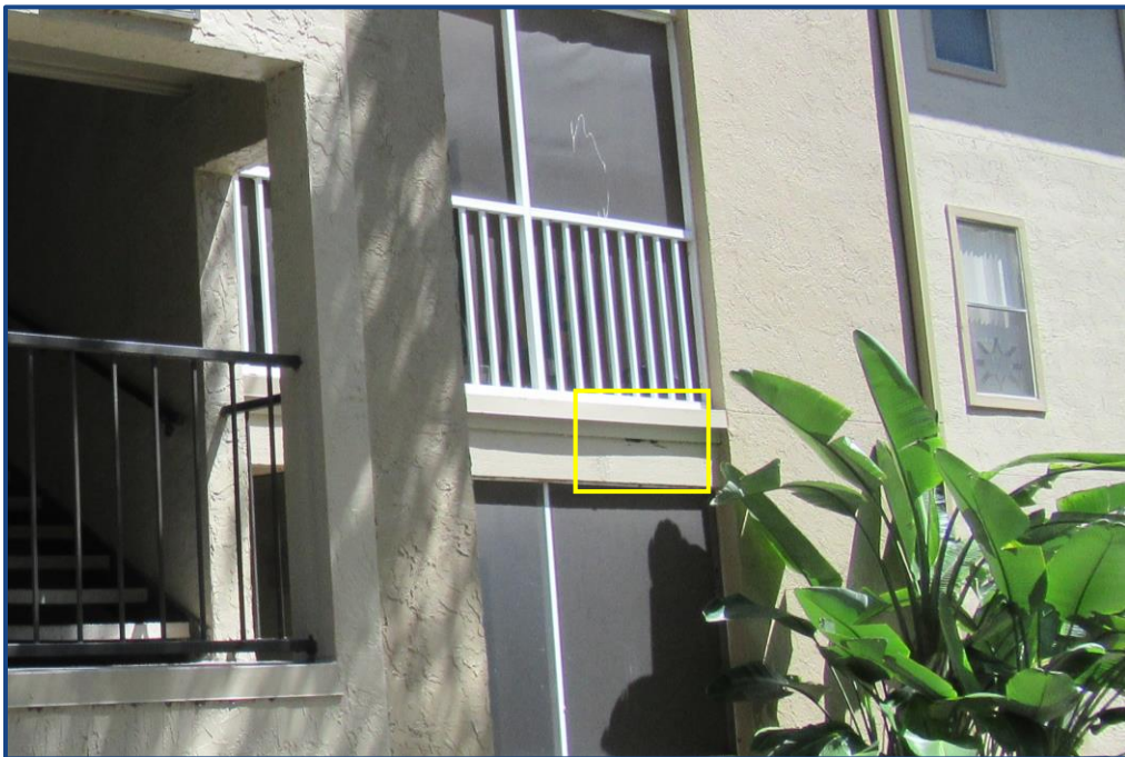
Photograph No. 10: Damage to the wood beam located at the balcony edge of Unit 201.
