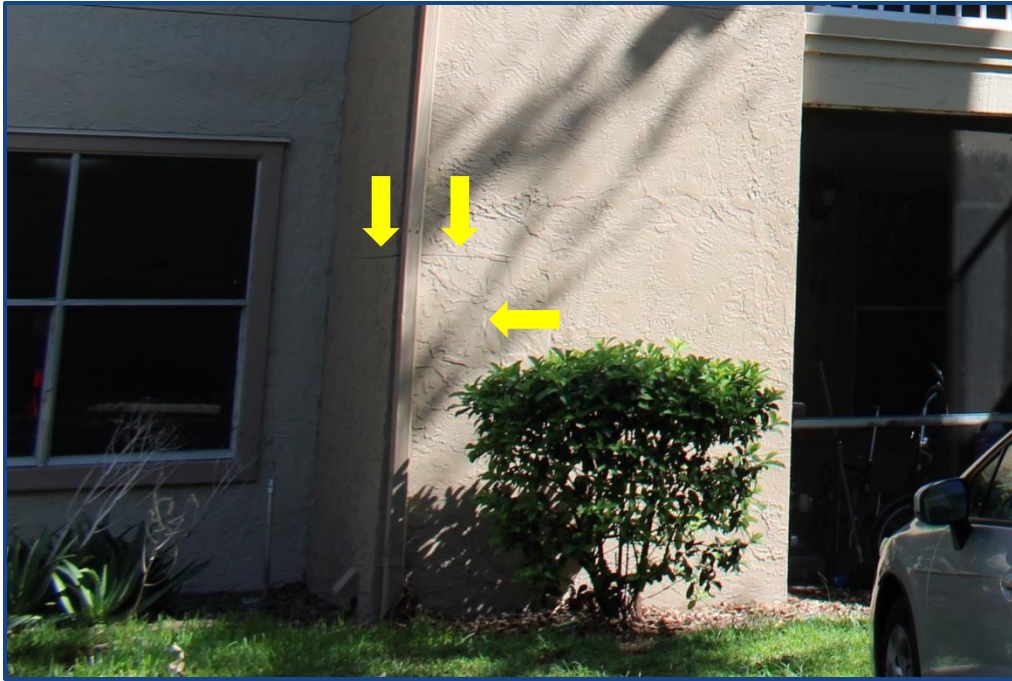
Photograph No. 15: Cracks in the exterior wall stucco finish located on the south side of the building.
