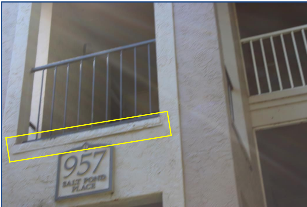
Photograph No. 12: Corrosion and damage to the metal flashing at the edge of the stairway landing slab at the north stairway.
