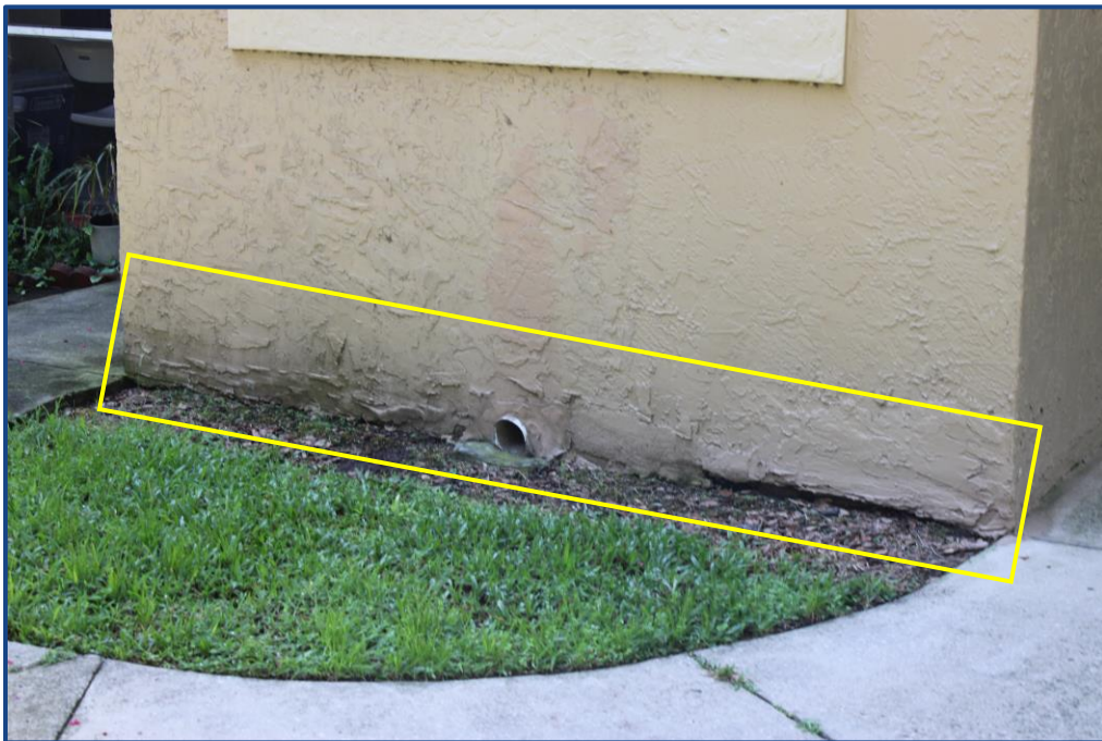
Photograph No. 14: Damage to the previously patched exterior wall stucco located at the drainage scupper in the north stairway.
