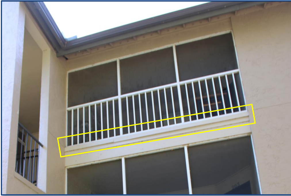
Photograph No. 11: Damage and separation to the metal flashing at the edge of the balcony slab on Unit 303.
