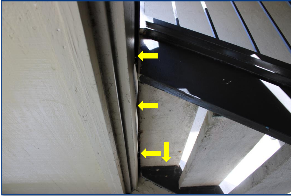
Photograph No. 17: Crack in a concrete step and separation of the steel framing from the stairway landing slab located in the south stairway.
