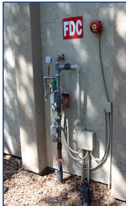
Photograph No. 20: Fire riser system and fire alarm.
