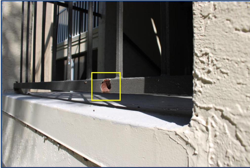
Photograph No. 19: Damage and corrosion to the metal guardrail located in the south stairway.
