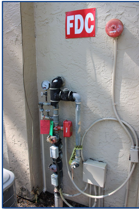
Photograph No. 21: Fire riser system and fire alarm.
