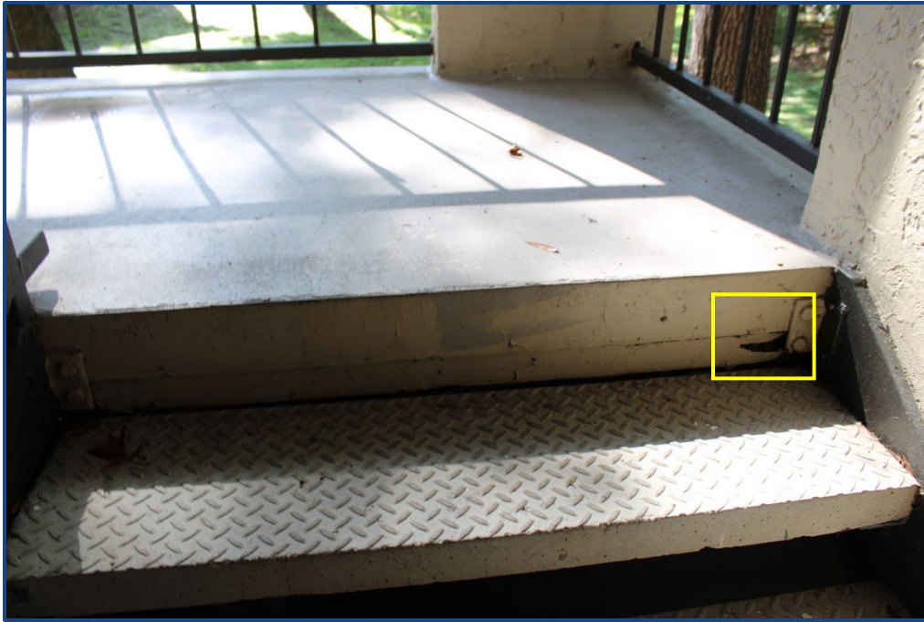
Photograph No. 11: Damage to the wood beam at the stairway landing located in the east stairway.
