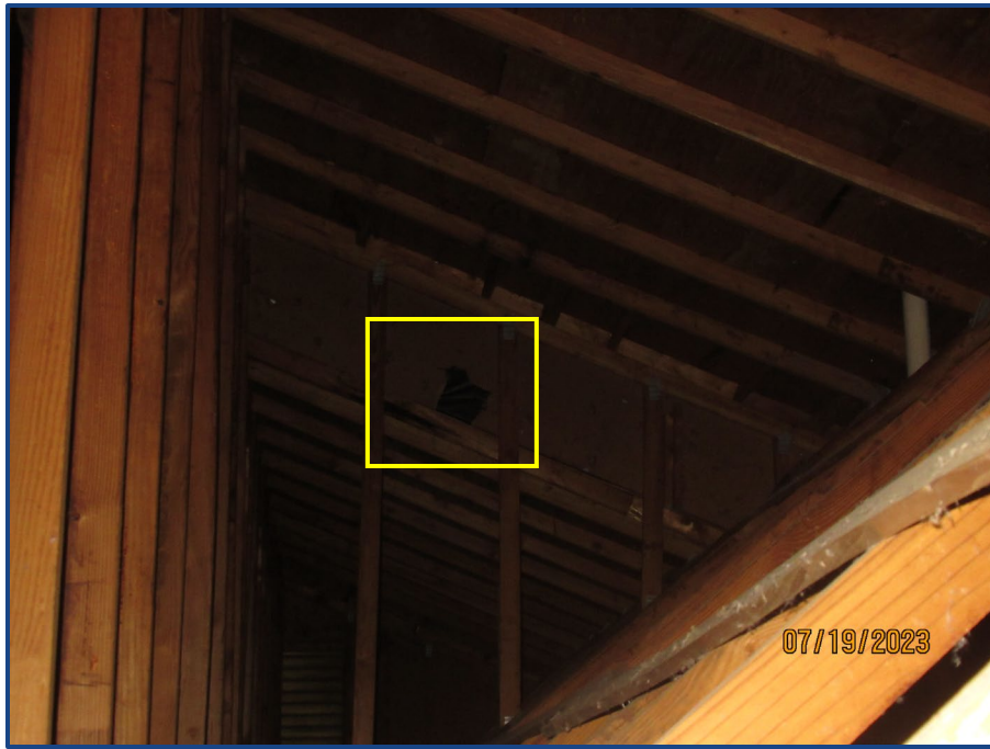
Photograph No. 9: Hole in the plywood wall sheathing located in the attic.
