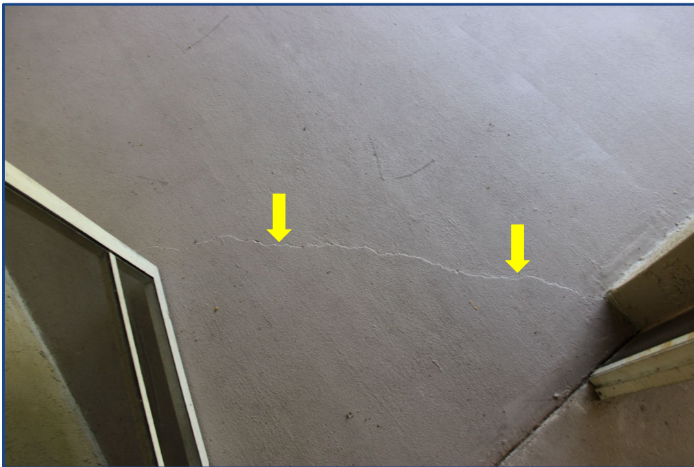
Photograph No. 16: Crack in the concrete balcony slab on Unit 303.
