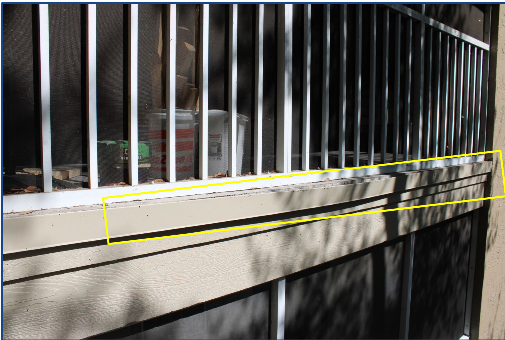
Photograph No. 12: Corrosion and separation of the metal flashing at the edge of the balcony slab on Unit 203.
