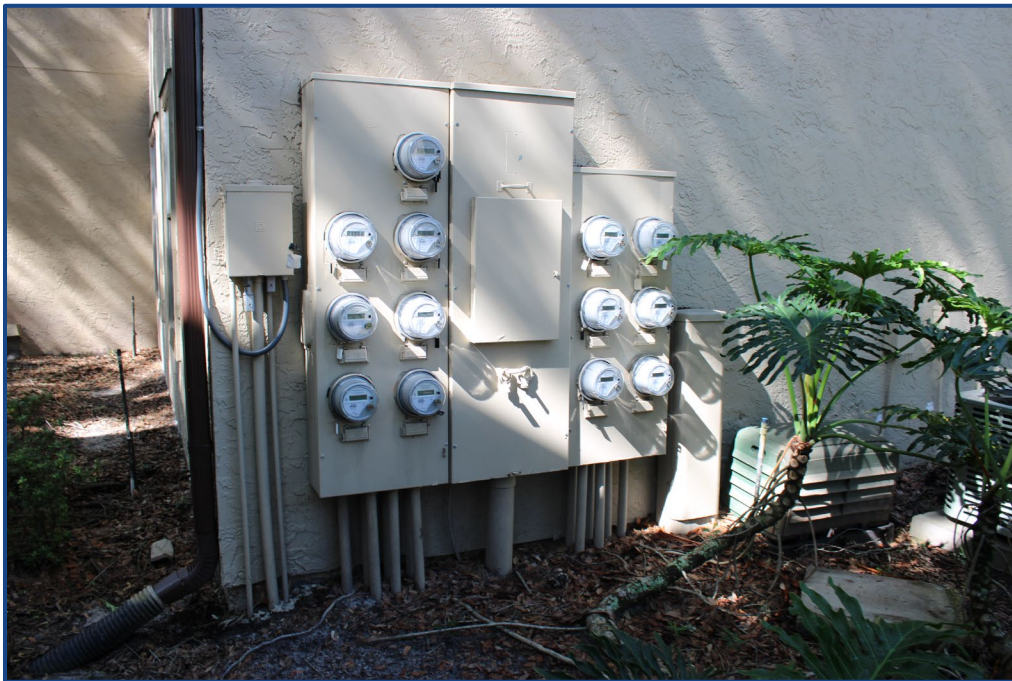
Photograph No. 20: Electrical meters.
