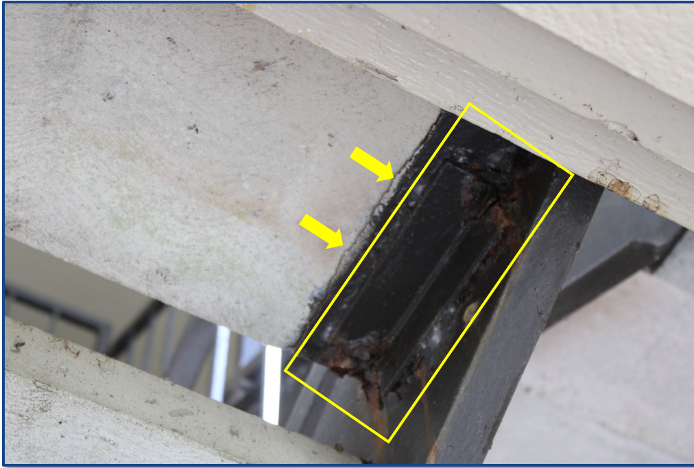
Photograph No. 17: Crack in a concrete step and corrosion to the steel framing located in the west stairway.
