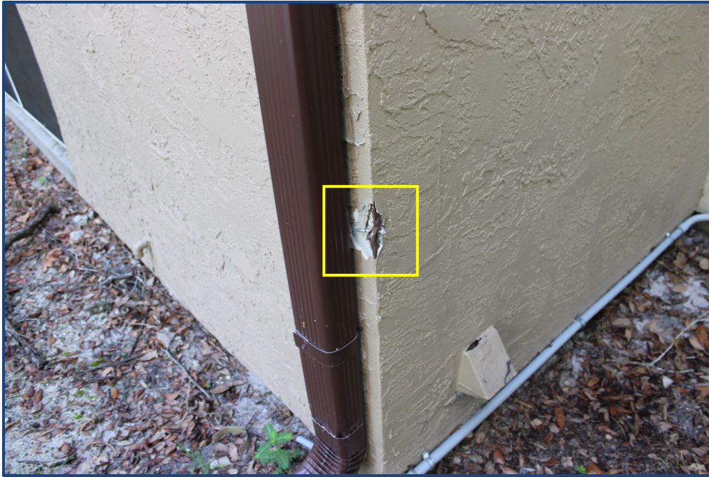
Photograph No. 15: Damage to the exterior wall stucco finish located at the west side of the building.
