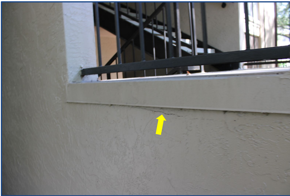
Photograph No. 14: Crack in the exterior wall stucco finish located on the east stairway.
