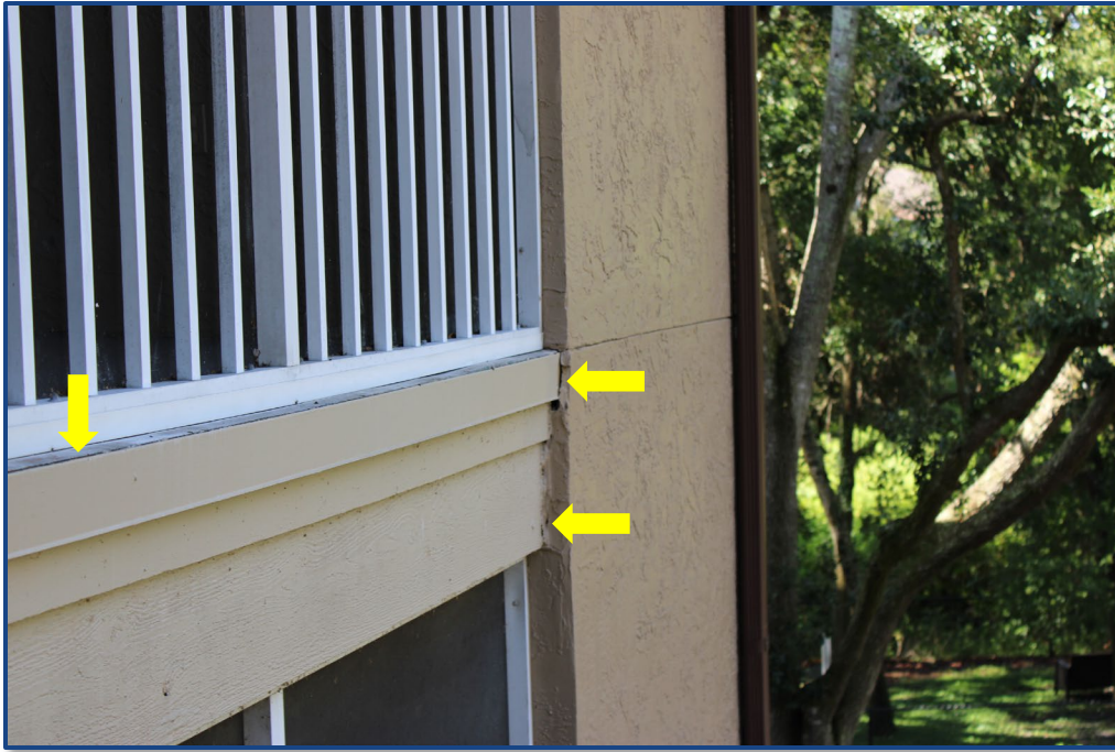
Photograph No. 13: Cracks in the stucco wall finish and separation of the metal flashing at the edge of the balcony slab on Unit 303.
