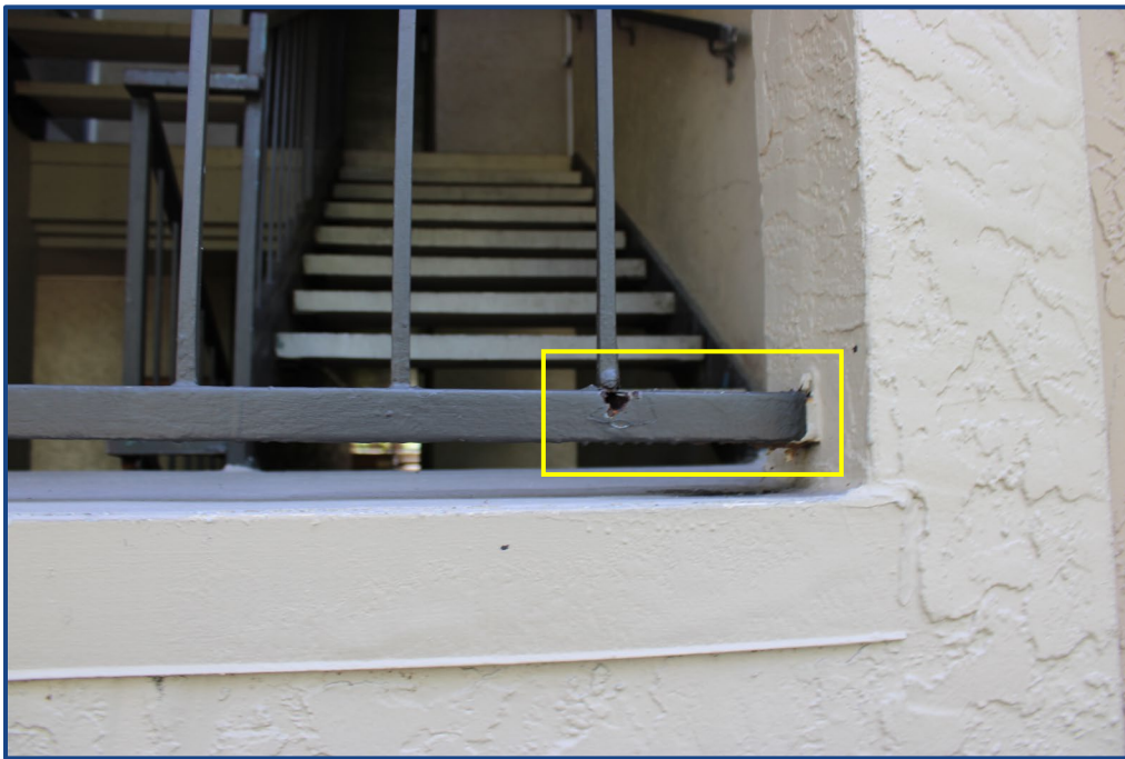
Photograph No. 18: Corrosion to the metal guardrail located in the west stairway.
