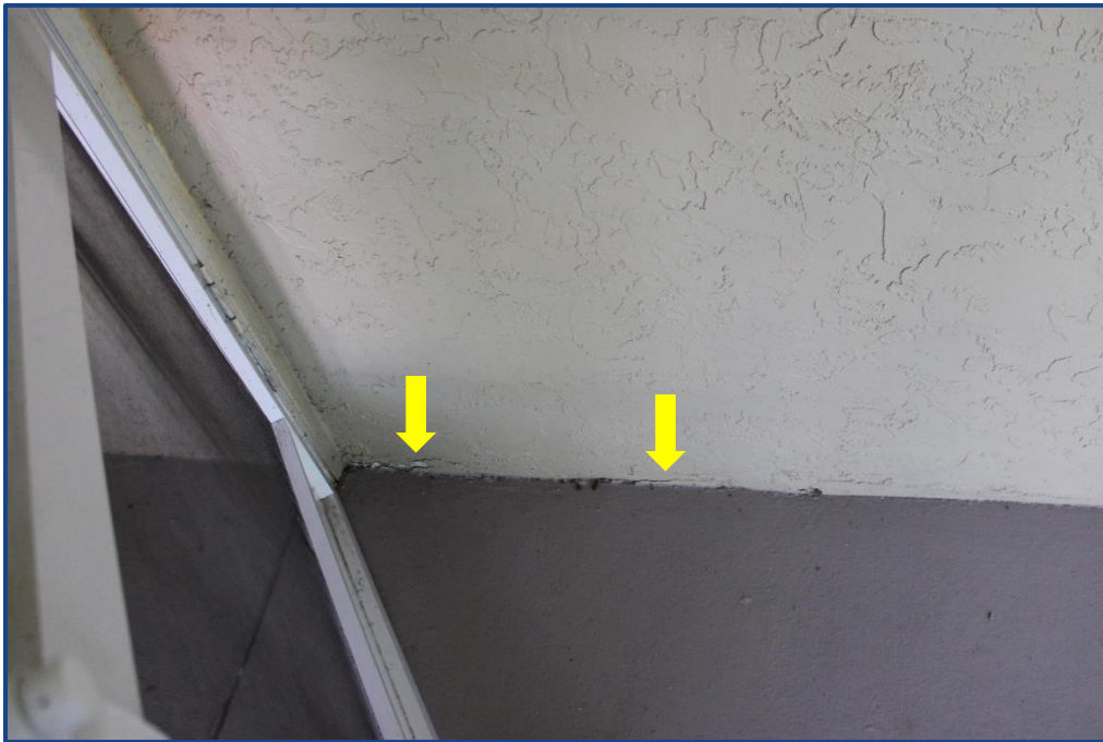
Photograph No. 10: Cracks in the exterior wall stucco finish located on Unit 203.
