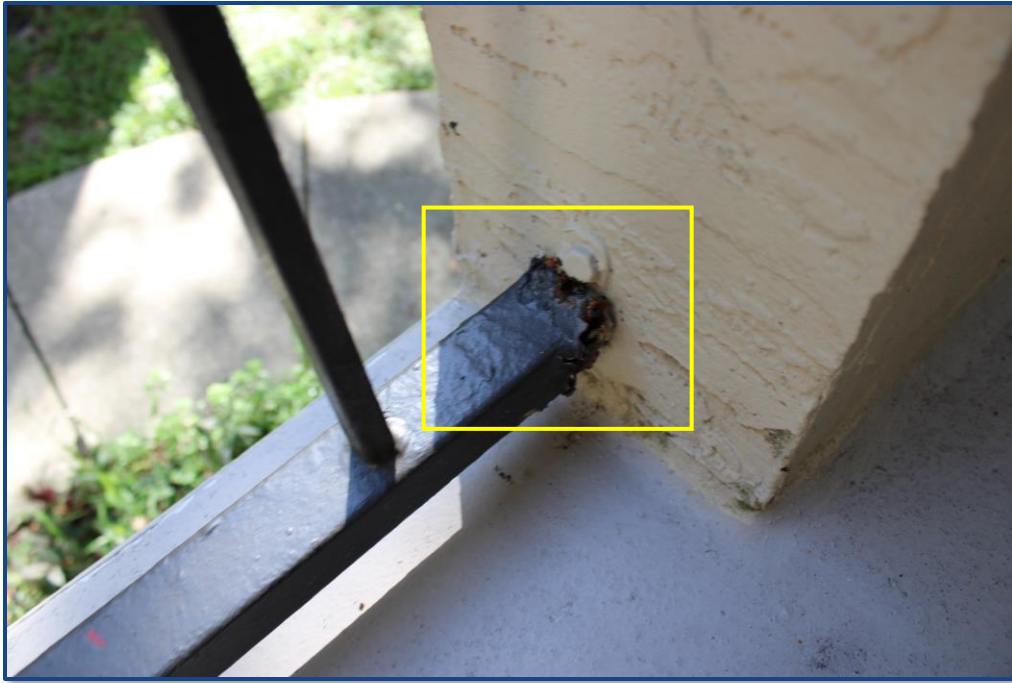
Photograph No. 17: Corrosion to the metal guardrail located in the east stairway.
