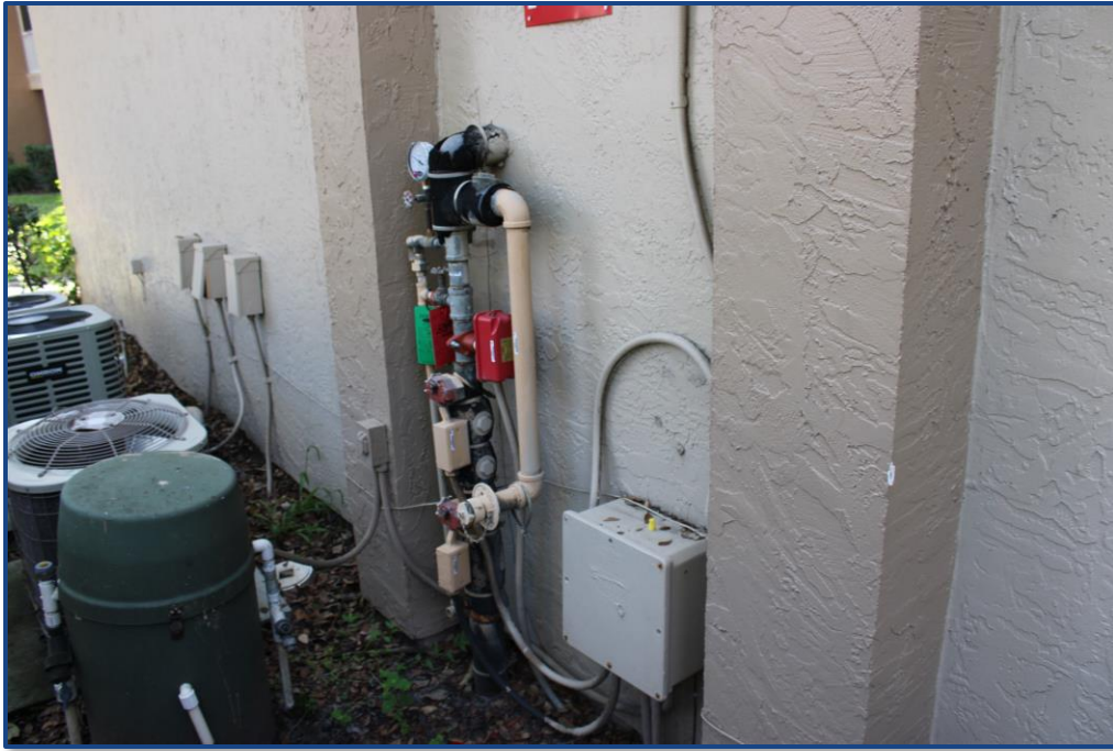
Photograph No. 19: Fire riser system.
