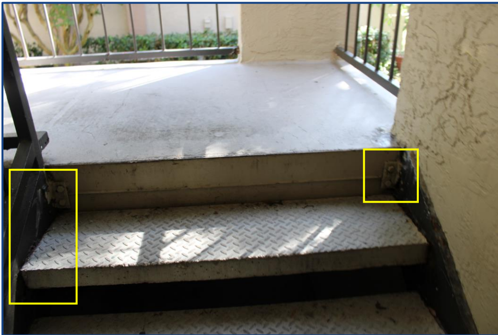
Photograph No. 14: Corrosion to the steel framing located in the east stairway.
