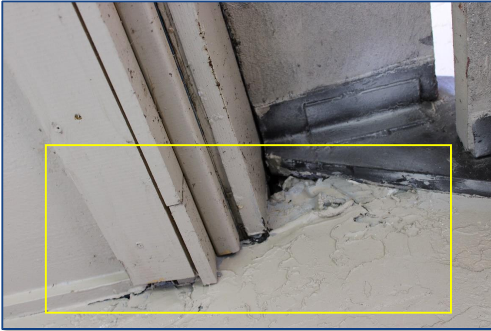
Photograph No. 9: Damage and previous patch to the exterior wall stucco finish located in the east stairway.
