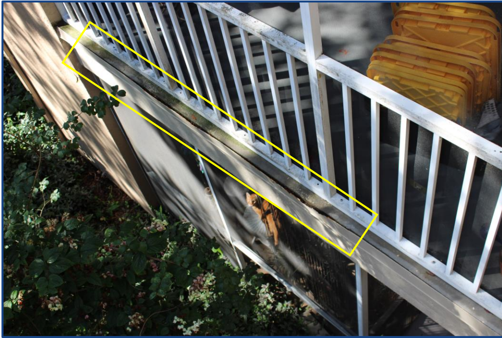
Photograph No. 11: Cracks in the balcony slab and corrosion and separation of the metal flashing at the edge of the balcony slab on Unit 202.
