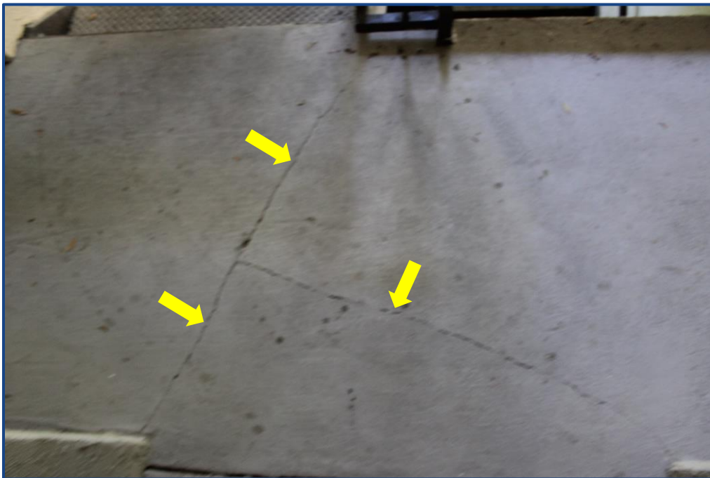
Photograph No. 12: Cracks in the concrete slab located on the 2nd floor.
