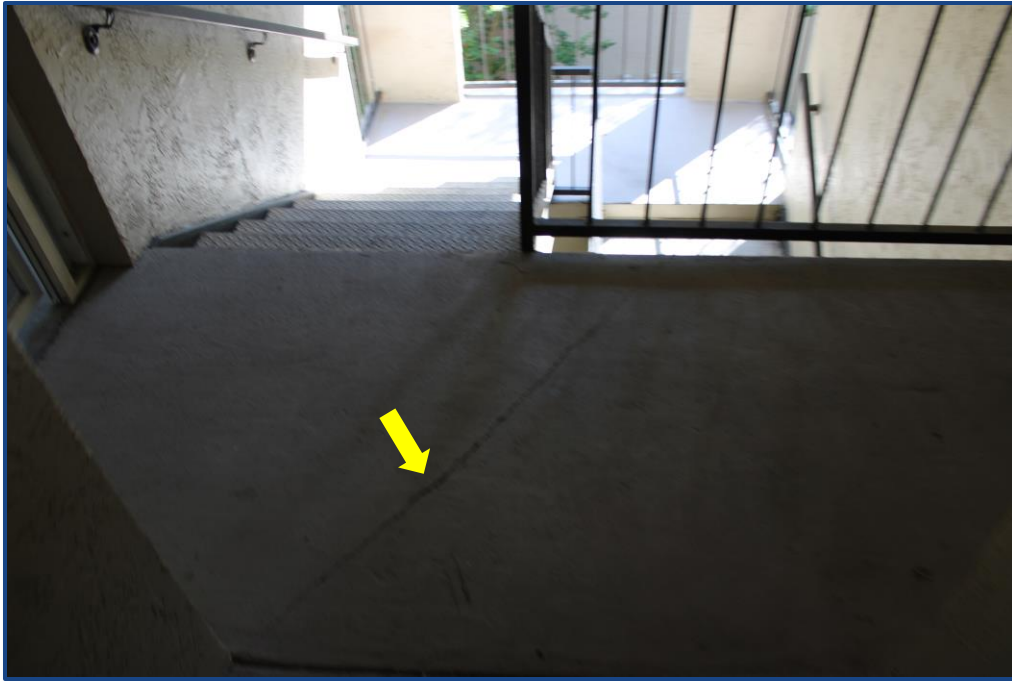
Photograph No. 13: Crack in the concrete slab located on the 3rd floor.
