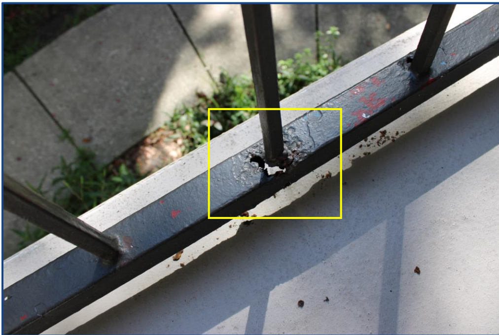
Photograph No. 16: Corrosion to the metal guardrail located in the east stairway.
