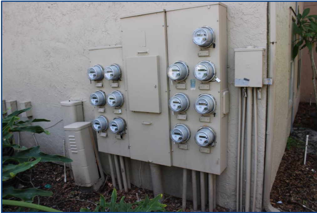
Photograph No. 18: Electrical meters.
