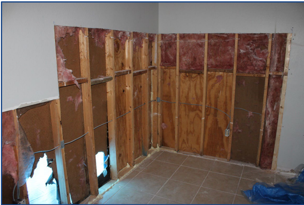
Photograph No. 20: View of the wood framing fire damage repairs located in Unit 201.
