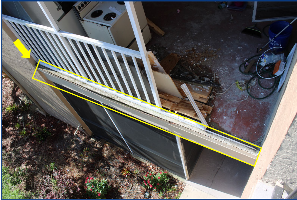
Photograph No. 11: Crack in the stucco wall finish, damage to the metal flashing at the edge of the balcony slab, and damaged balcony railing on Unit 204.
