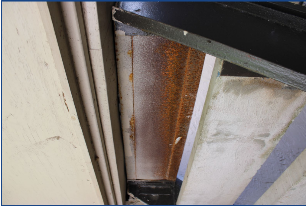
Photograph No. 17: Corrosion to the steel framing located in the north stairway.
