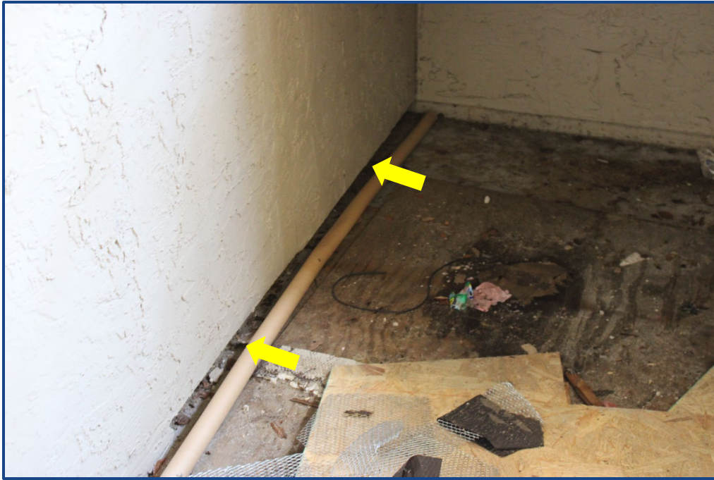
Photograph No. 13: Damage to the exterior wall stucco finish located in the north stairway.
