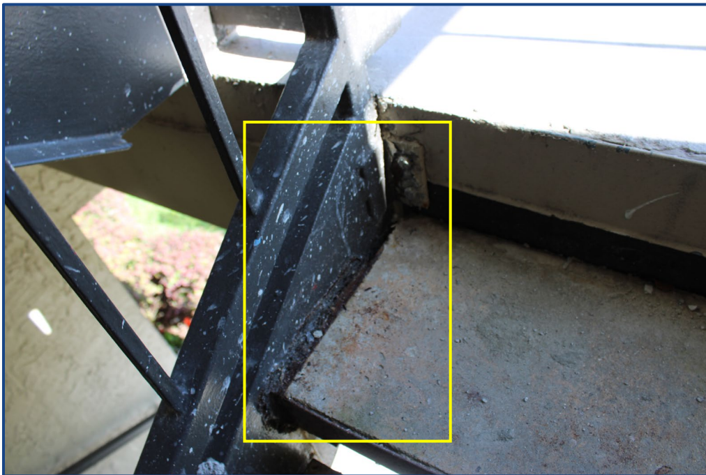
Photograph No. 16: Corrosion to the steel framing located in the north stairway.
