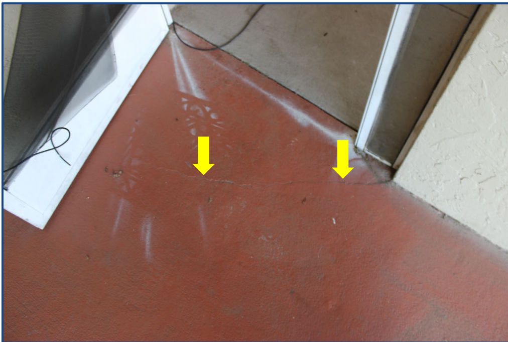
Photograph No. 14: Crack in the balcony slab on Unit 304.
