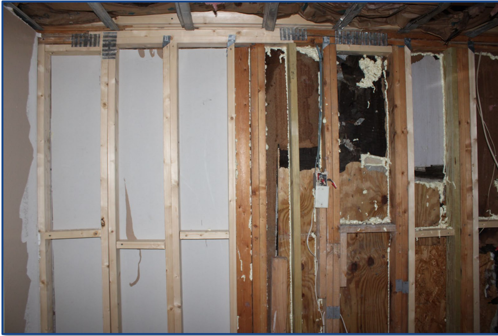
Photograph No. 19: View of the wood framing fire damage repairs located in Unit 101.
