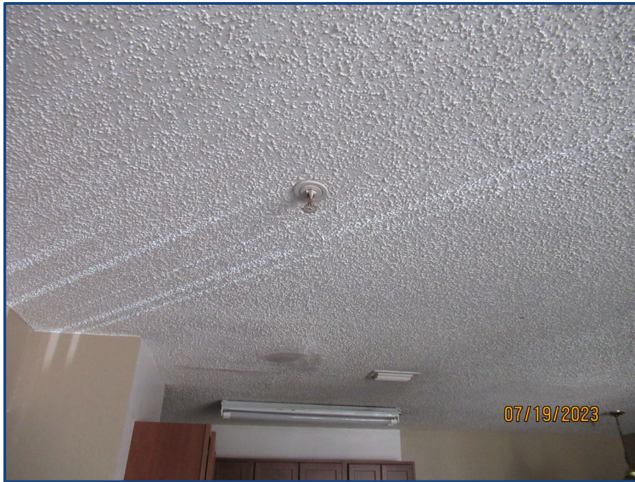
Photograph No. 23: Fire sprinkler head in Unit 101.
