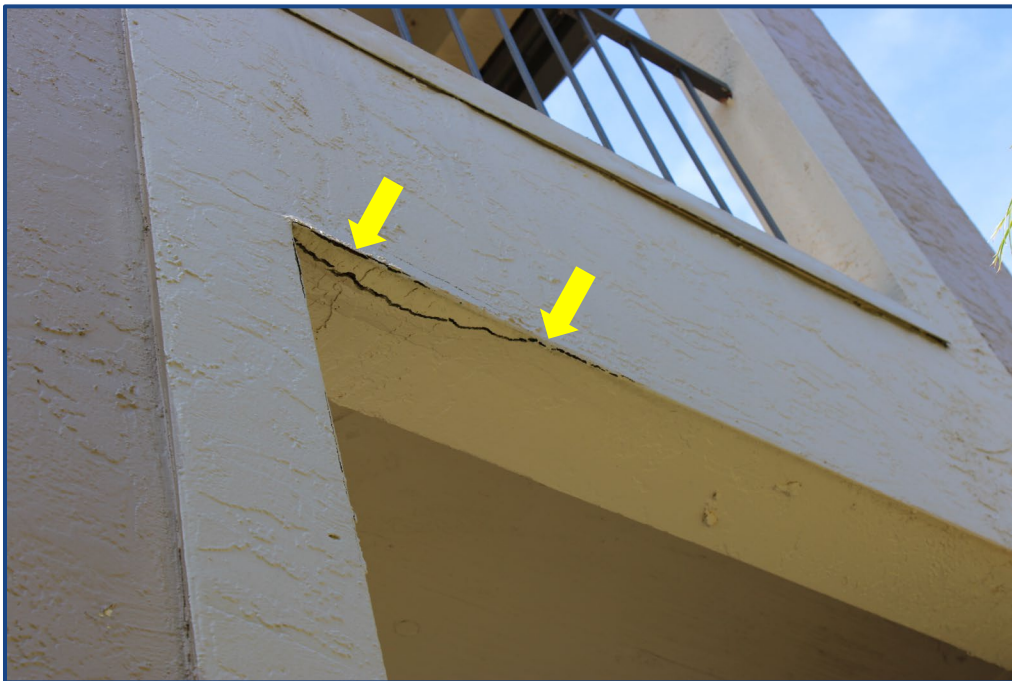
Photograph No. 12: Cracks in the exterior wall stucco finish located on the north stairway.
