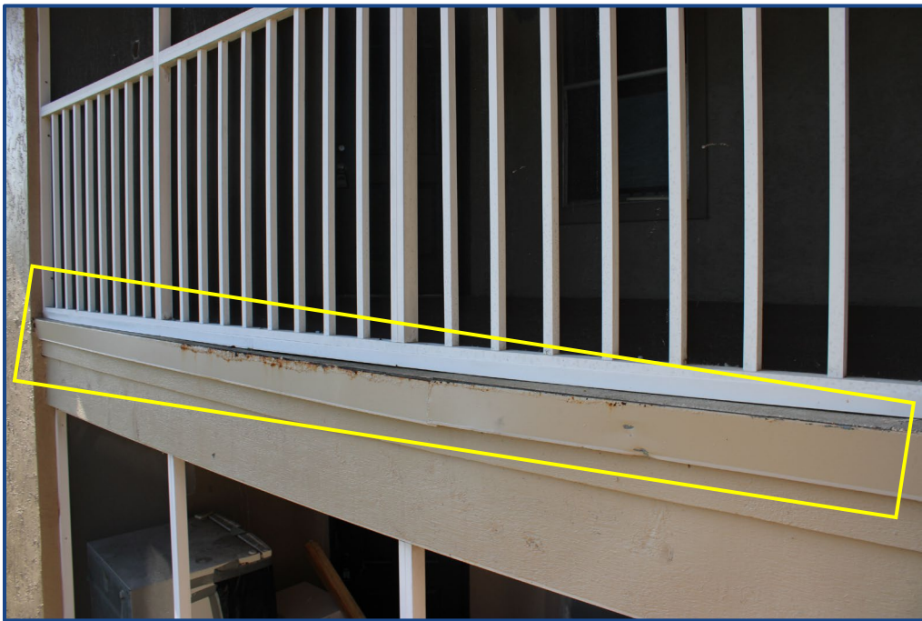
Photograph No. 10: Corrosion and separation of the metal flashing at the edge of the balcony slab on Unit 304.
