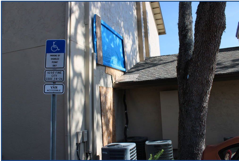
Photograph No. 21: View of the fire damaged areas on Unit 101 and 201 from the exterior.
