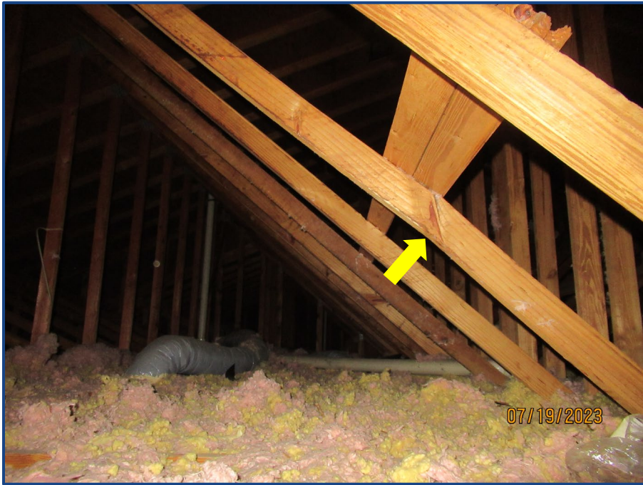
Photograph No. 8: View of a broken prefabricated wooden roof truss member.
