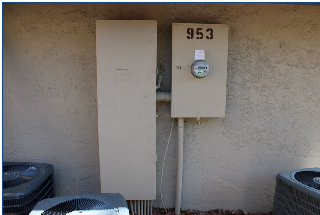
Photograph No. 22: Electrical meter and electrical panel.
