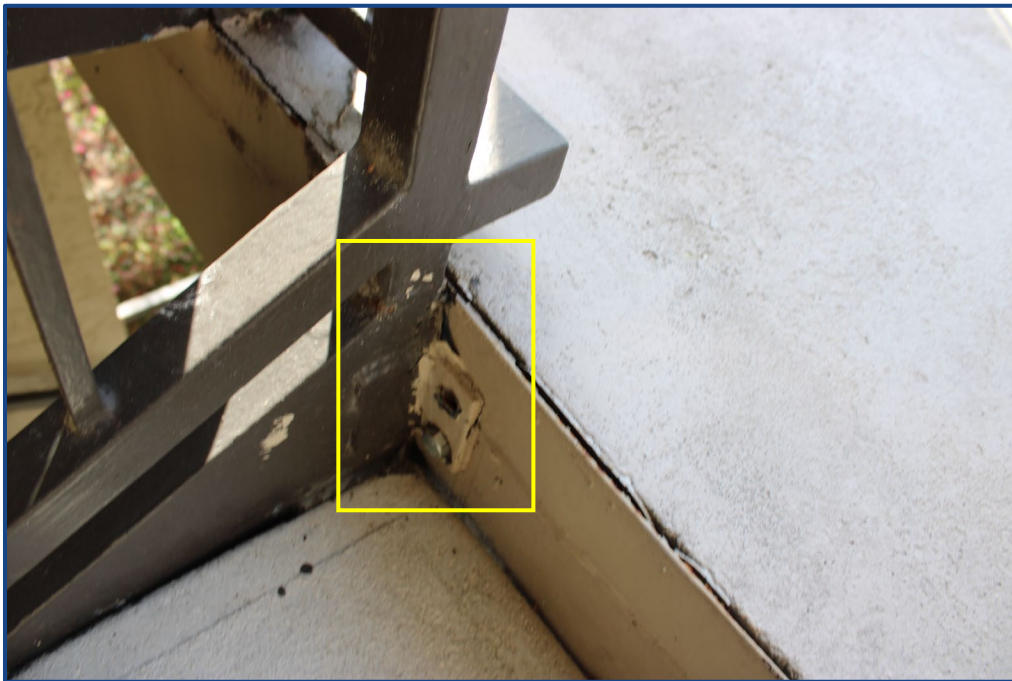
Photograph No. 14: Missing bolt and corrosion to the steel framing located in the southeast stairway.
