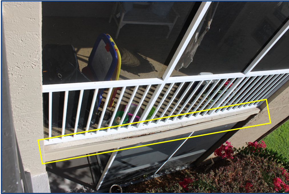
Photograph No. 9: Cracks in the balcony slab and corrosion and separation of the metal flashing at the edge of the balcony slab on Unit 203.
