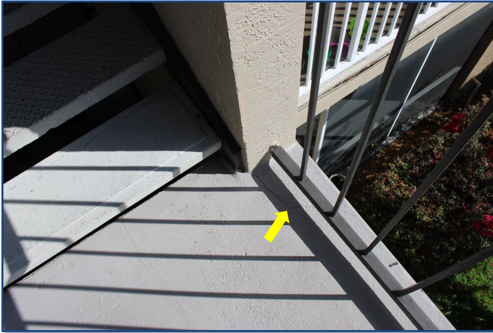
Photograph No. 13: Crack in the stairway landing in the southeast stairway.
