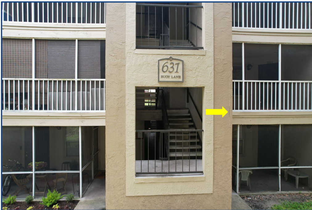
Photograph No. 10: Crack in the exterior wall stucco finish.
