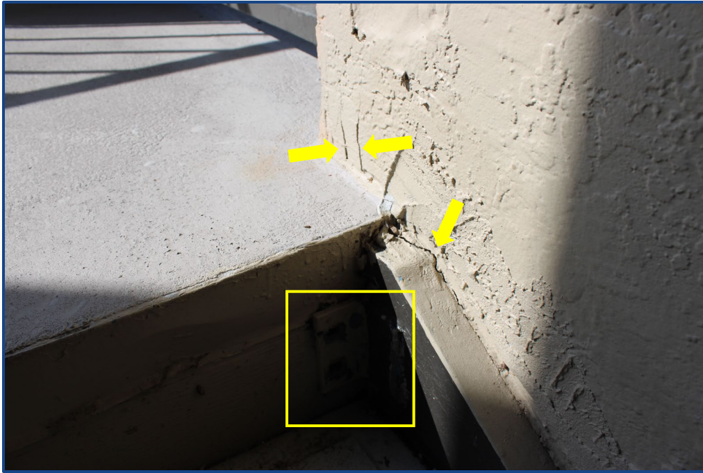
Photograph No. 15: Missing fastener, cracks in the stucco and corrosion to the steel framing located in the southeast stairway.
