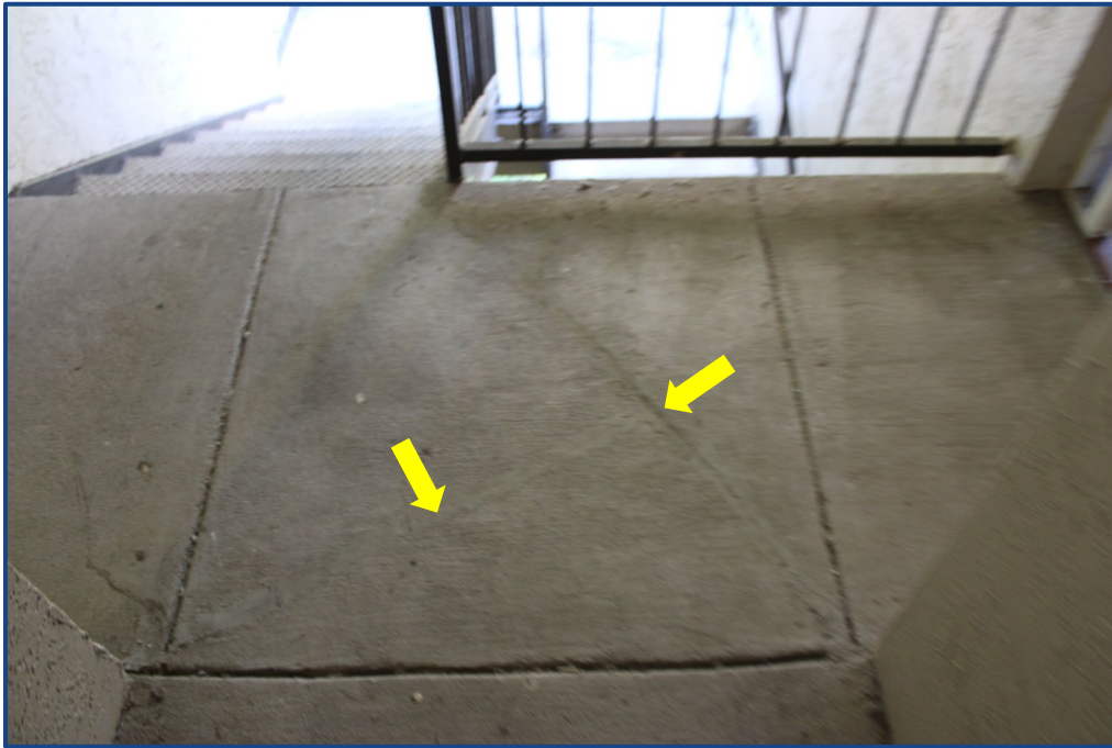
Photograph No. 12: Previously sealed cracks in the concrete slab located on the 3rd floor.
