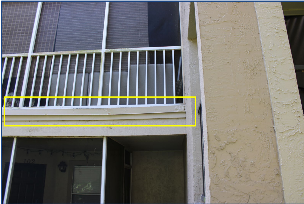
Photograph No. 8: Corrosion and separation of the metal flashing at the edge of the balcony slab on Unit 201.
