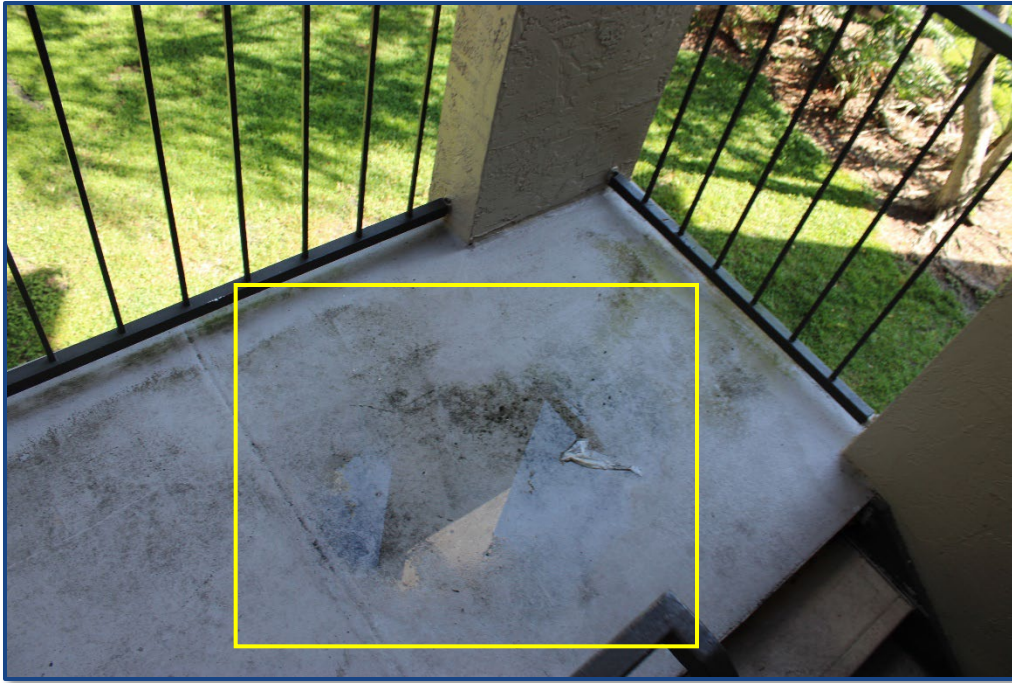
Photograph No. 11: Ponding on the stairway landing in the northwest stairway.
