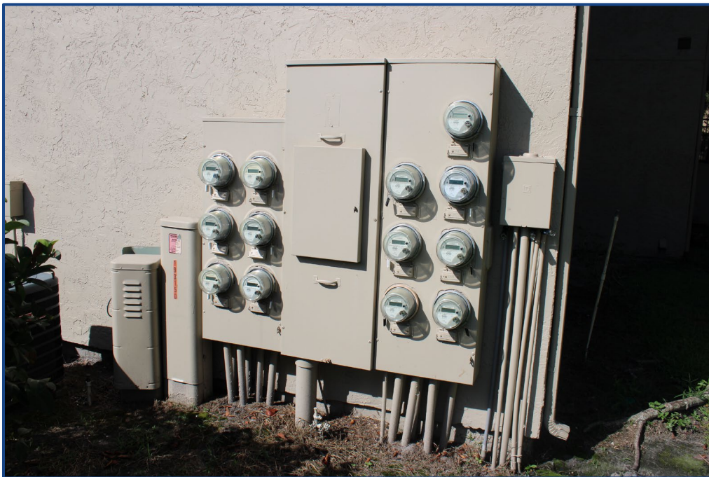
Photograph No. 16: Electrical meters.
