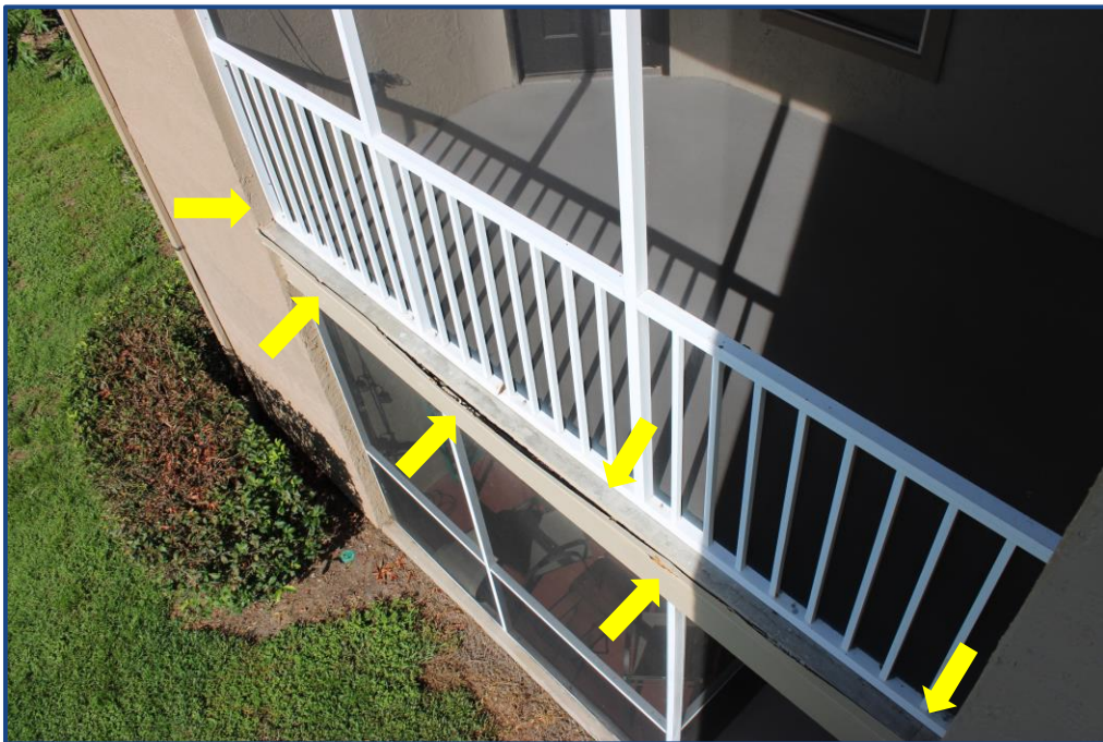
Photograph No. 14: Cracks in the stucco wall finish, cracks in the balcony slab, and damage to the metal flashing at the edge of the balcony slab on Unit 208.
