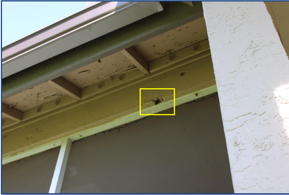
Photograph No. 11: Damage to the wood balcony framing located at the balcony on Unit 308.
