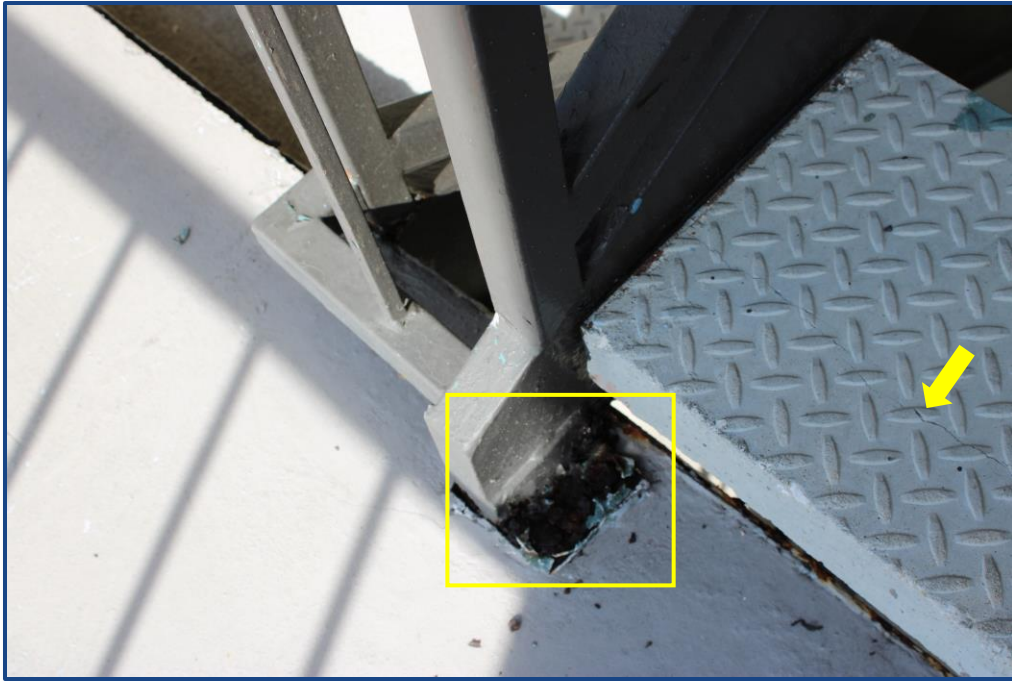
Photograph No. 23: Corrosion to the steel framing and crack in the concrete step located in the southeast stairway.
