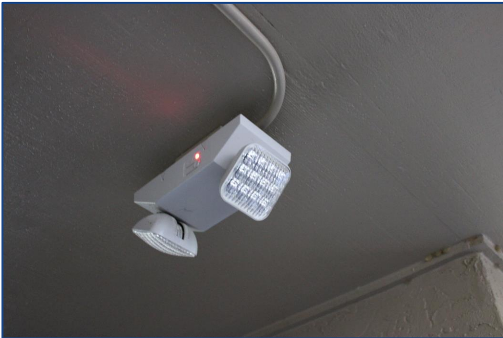
Photograph No. 26: Emergency lighting.
