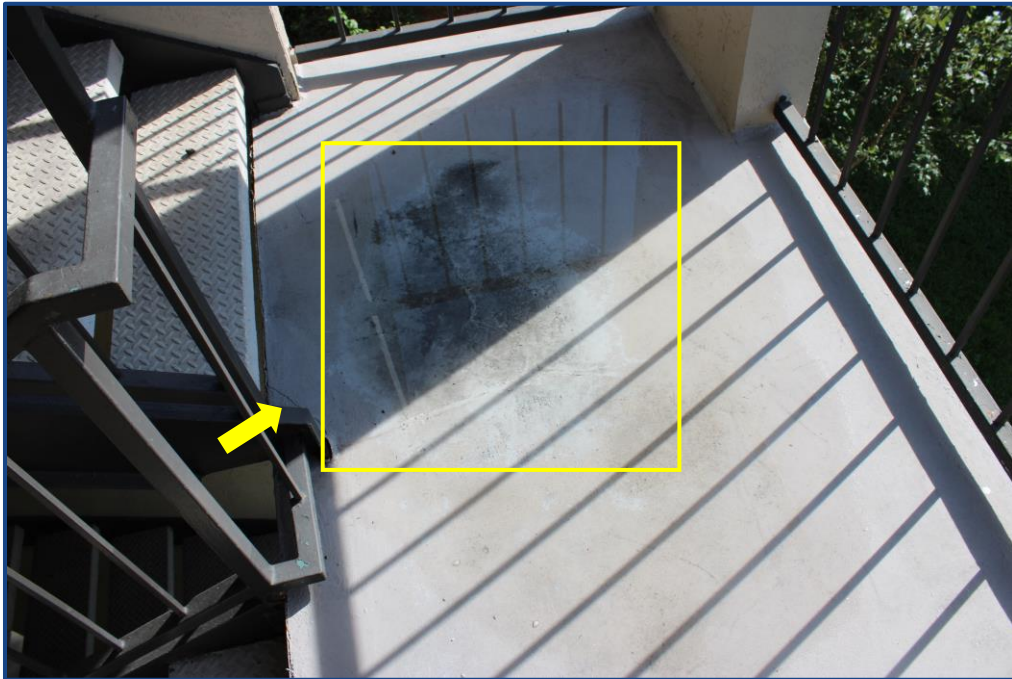
Photograph No. 18: Crack and ponding on the stairway landing in the northeast stairway.
