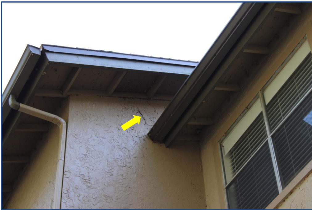
Photograph No. 16: Crack in the exterior wall stucco finish.
