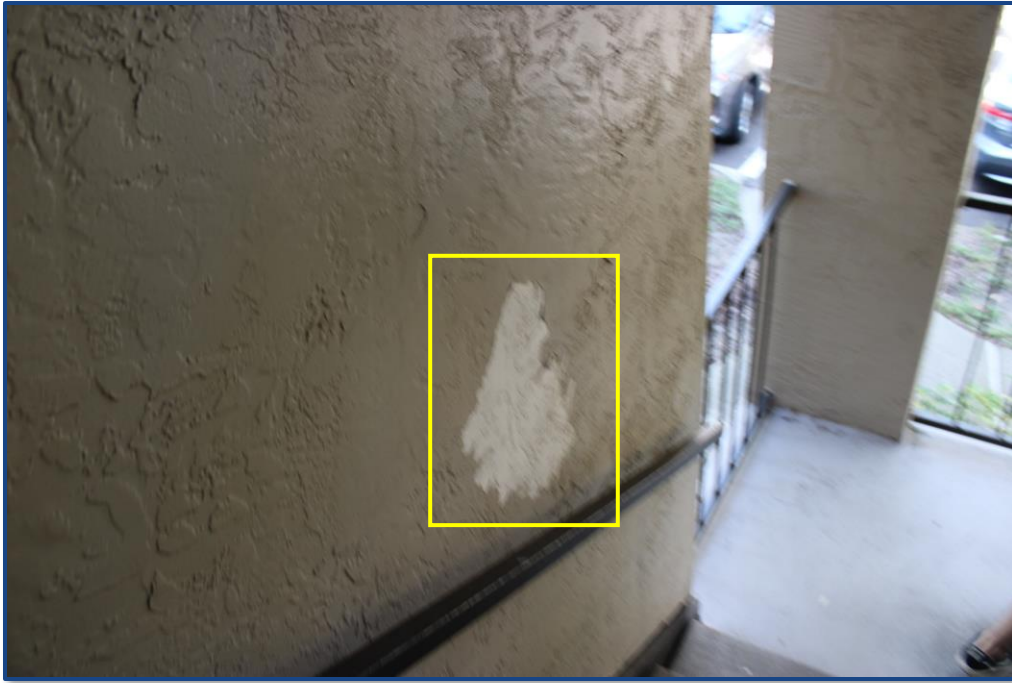
Photograph No. 17: Peeling paint located in the northwest stairway.
