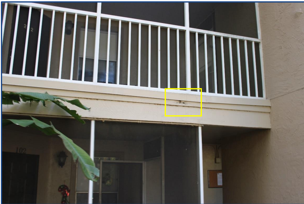
Photograph No. 12: Damage to the wood beam located at the balcony edge on Unit 202.
