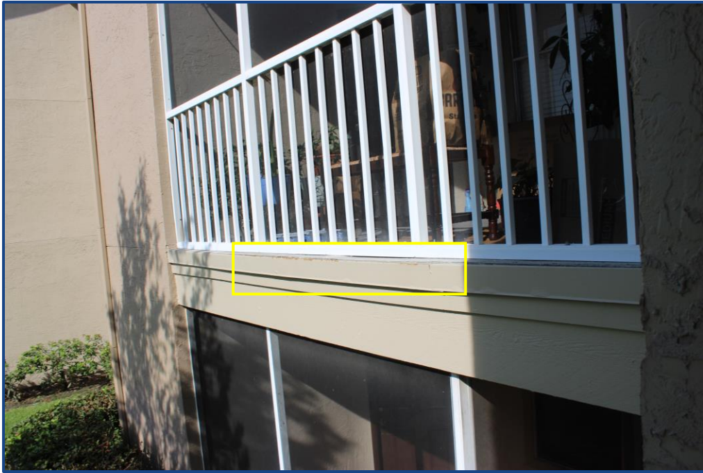
Photograph No. 13: Corrosion and separation of the metal flashing at the edge of the balcony slab on Unit 206.
