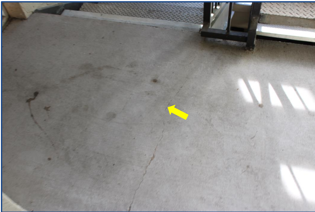
Photograph No. 20: Crack in the concrete slab located on the 2nd floor.
