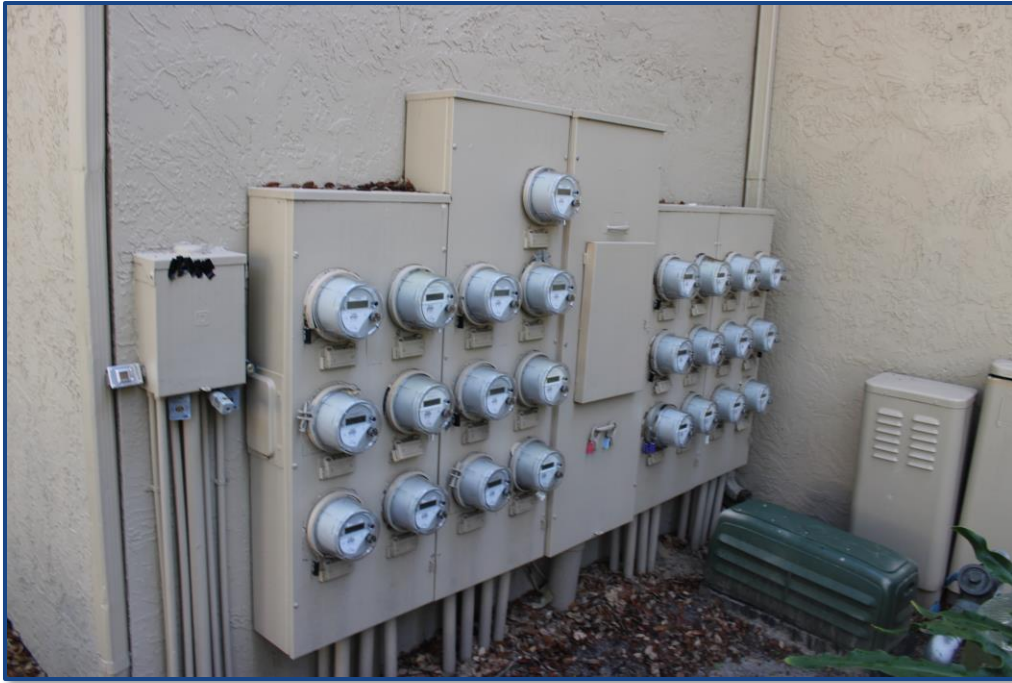
Photograph No. 25: Electrical meters.
