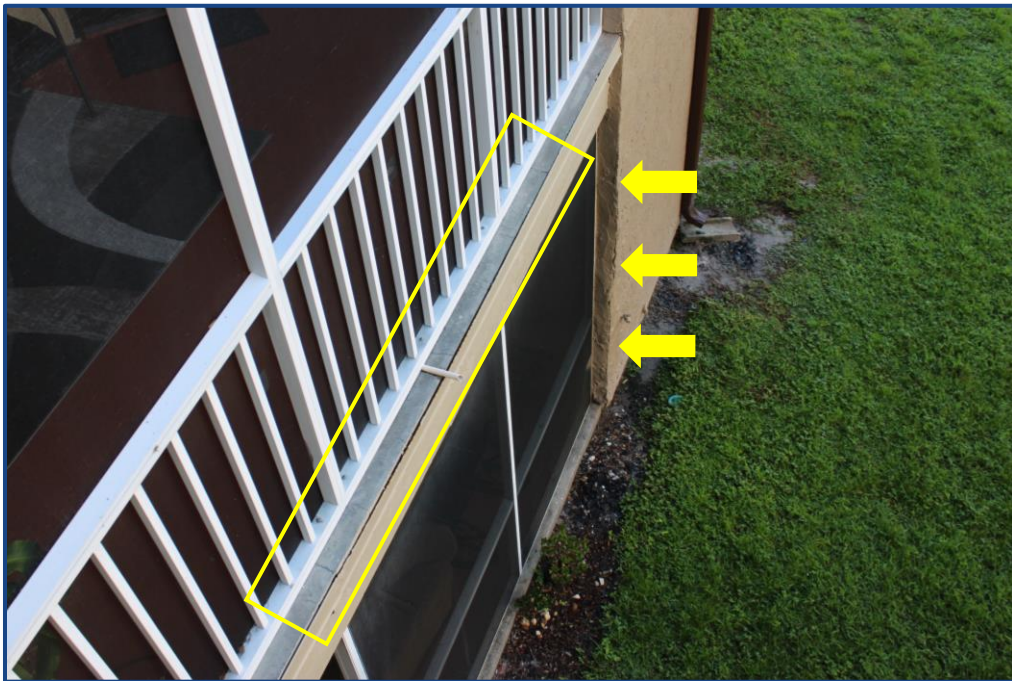
Photograph No. 16: Cracks in the exterior balcony slab on Unit 201 and cracks in the stucco finish at the 1st floor level.
