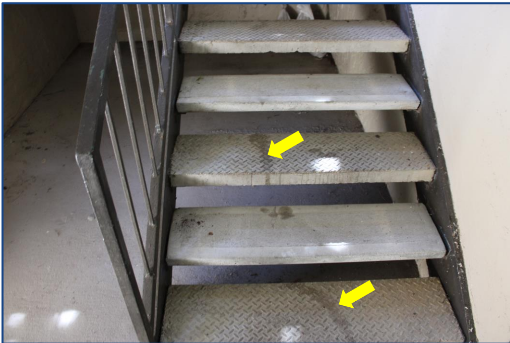
Photograph No. 18: Previously sealed cracks located in the concrete steps in the stairway.
