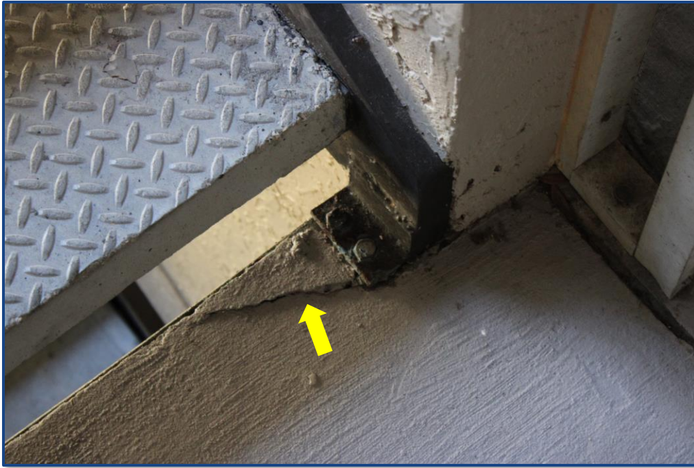
Photograph No. 15: Crack in the concrete slab located on the 2nd floor.
