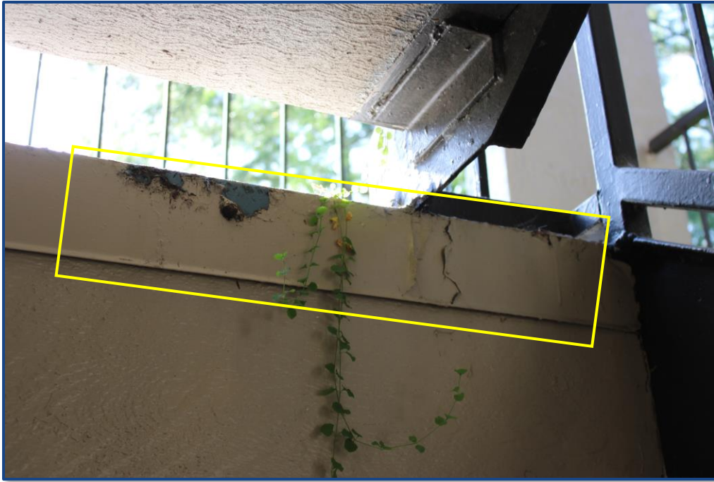
Photograph No. 17: Peeling of the paint finish and flora growth on the metal flashing located at the edge of the stairway landing slab.
