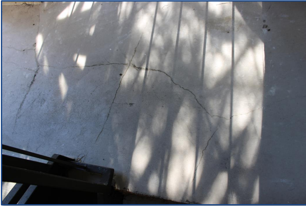
Photograph No. 11: Cracks in the concrete stairway landing.
