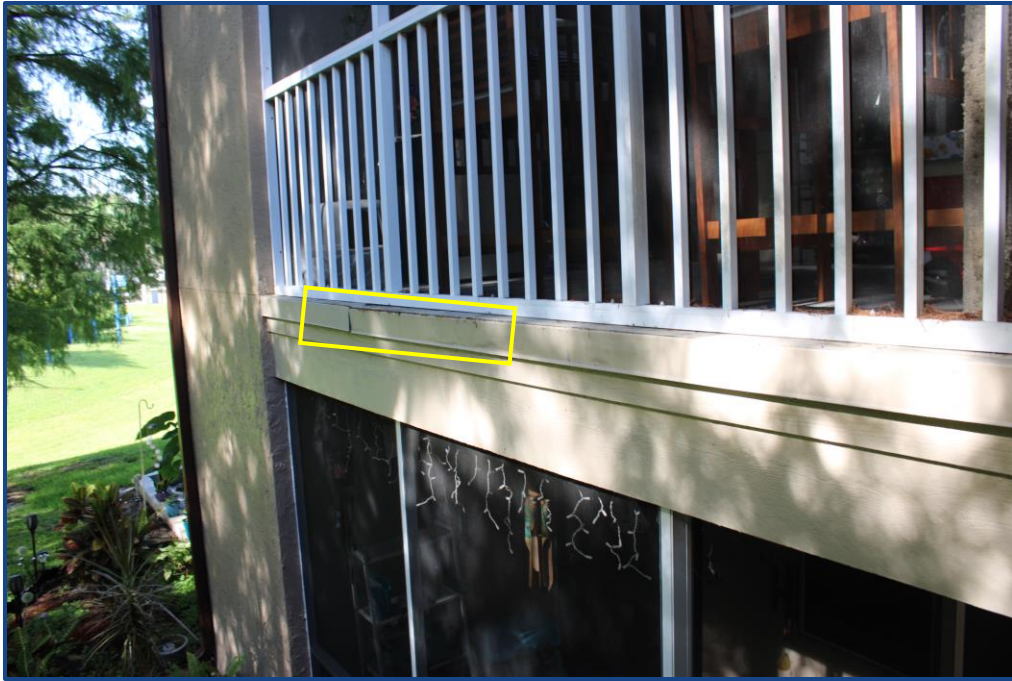
Photograph No. 13: Corrosion and separation of the metal flashing at the edge of the balcony slab on Unit 204.
