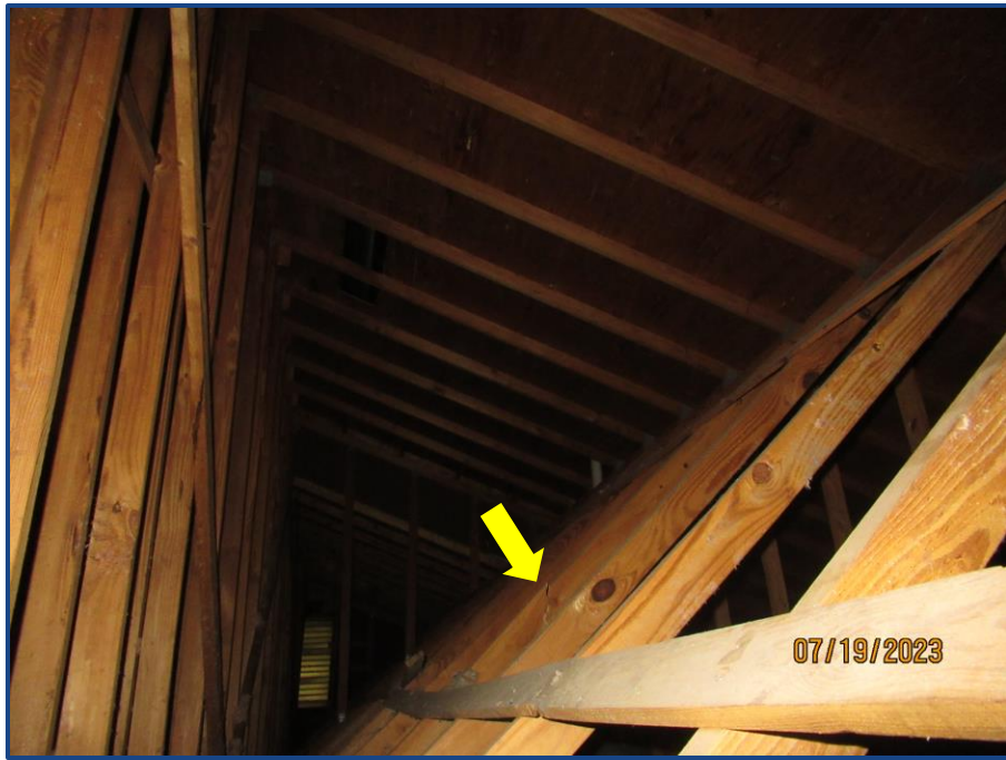
Photograph No. 7: View of a broken prefabricated wooden roof truss.
