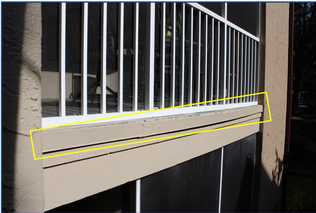
Photograph No. 14: Peeling and bubbling of the paint finish and separation of the metal flashing located at the edge of the balcony slab on Unit 203.
