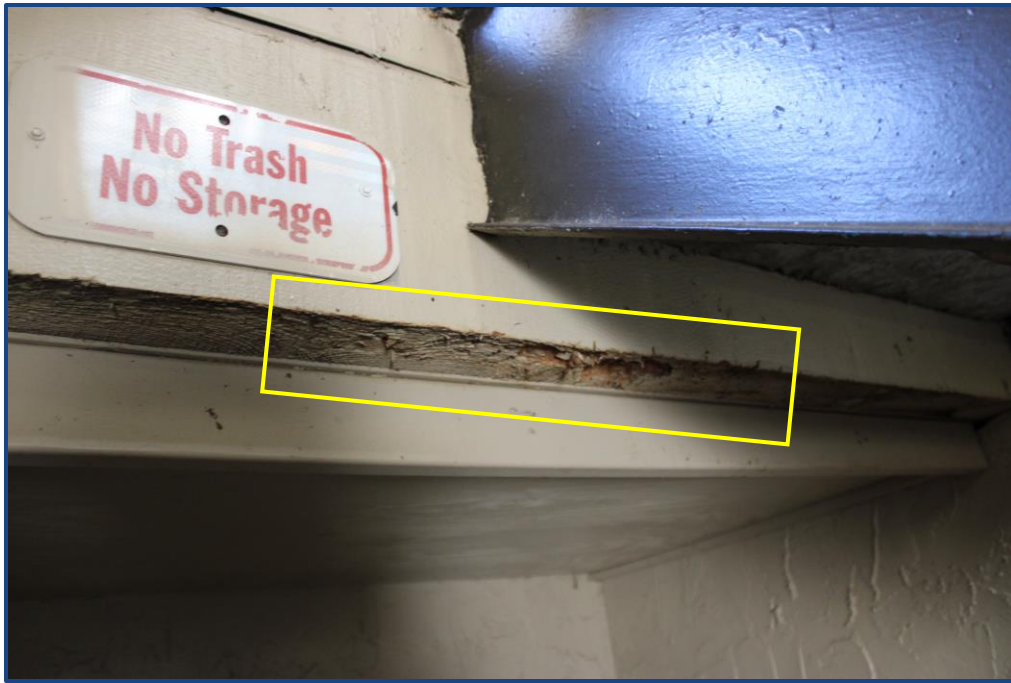
Photograph No. 9: Deterioration to the wood beam located at the 1st/2nd floor east stairway landing.
