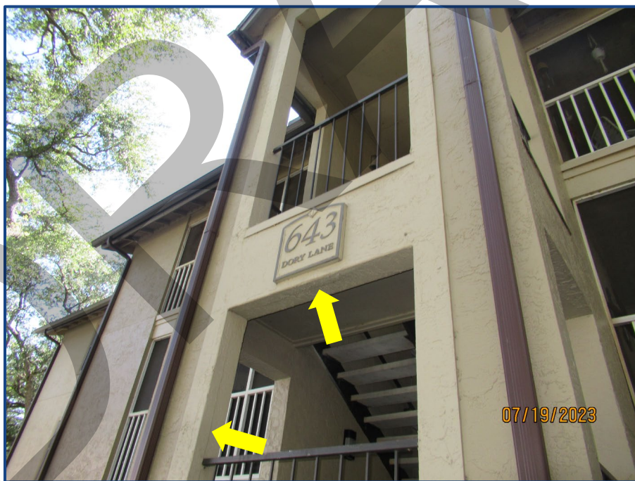
Photograph No. 10: Cracks in the exterior wall stucco finish located on the west stairway.
