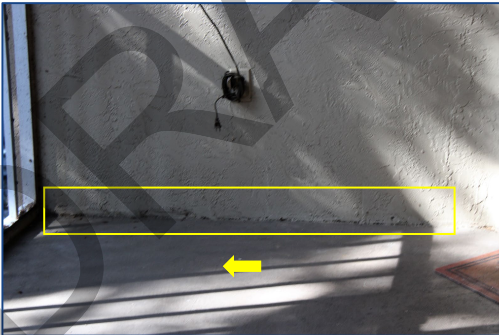
Photograph No. 12: Damage to the exterior wall stucco finish and crack in the balcony slab on Unit 204.
