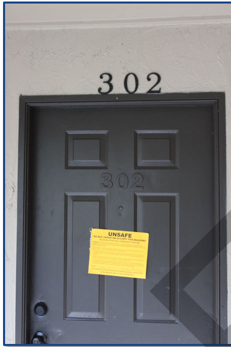
Photograph No. 17: Unsafe conditions declaration by order of the City of Altamonte Springs due to the broken fire sprinkler pipe in Unit 302.
