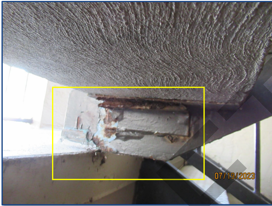
Photograph No. 13: Corrosion to the steel framing and metal flashing located in the west stairway.
