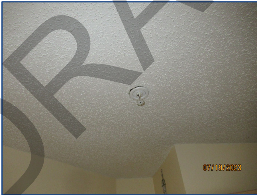
Photograph No. 18: Fire sprinkler head located in Unit 203.
