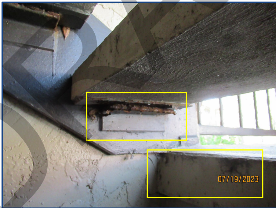
Photograph No. 14: Corrosion to the steel framing and metal flashing located in the west stairway.
