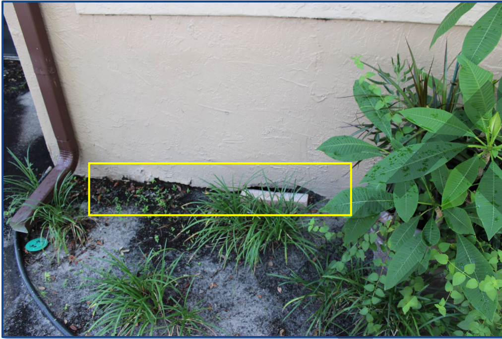
Photograph No. 11: Damage to the exterior wall stucco finish located on the west stairway.
