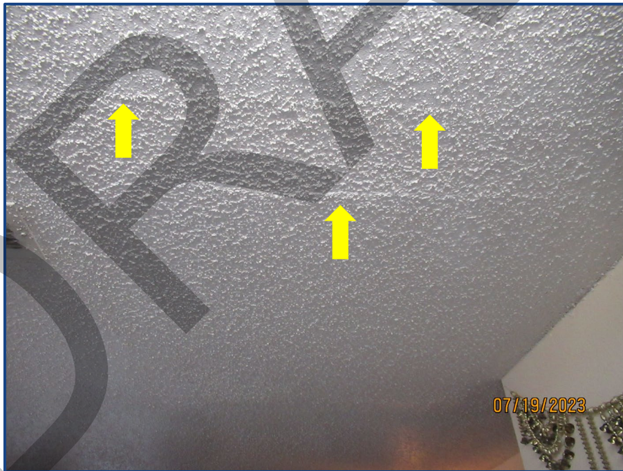
Photograph No. 16: Cracks in the ceiling in Unit 203 due to water leak.
