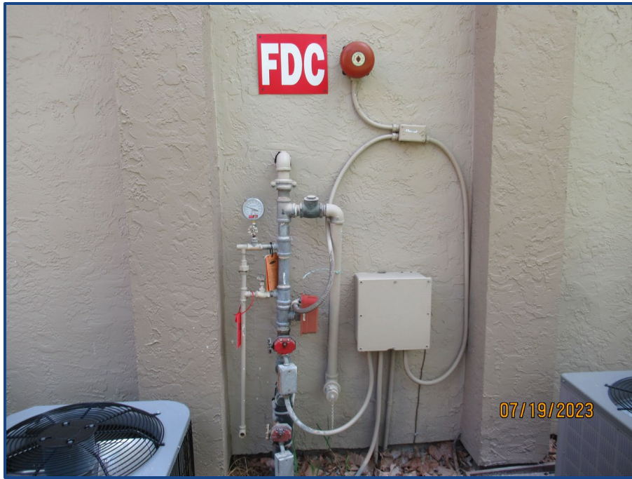
Photograph No. 21: Fire riser system and fire alarm.
