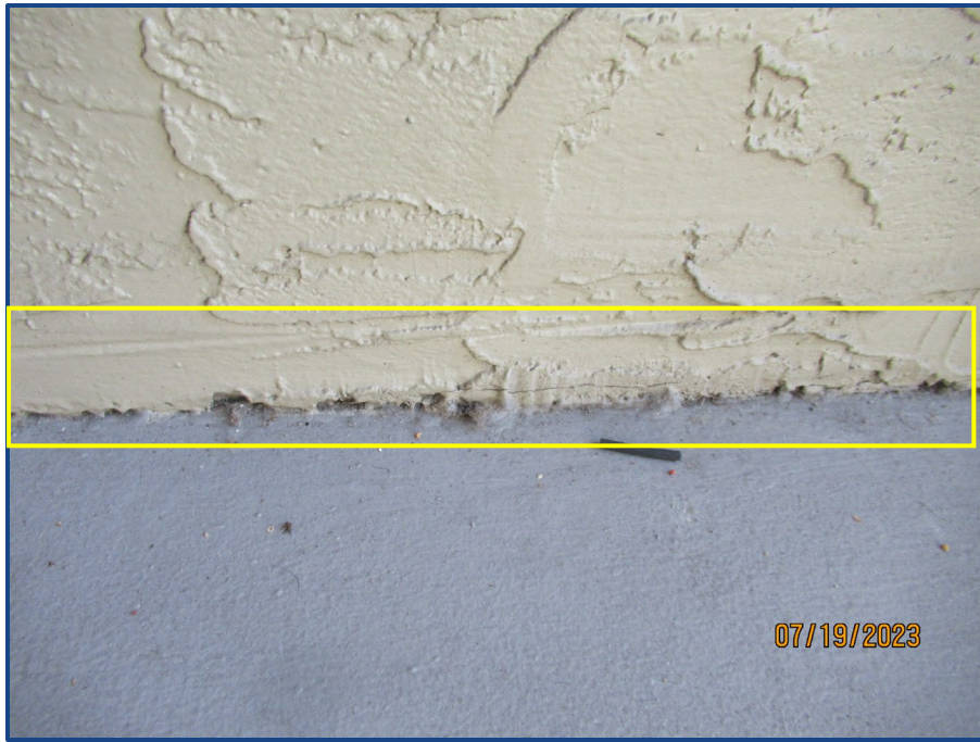
Photograph No. 15: Cracks and damage to the exterior wall stucco finish located on the balcony of Unit 206.
