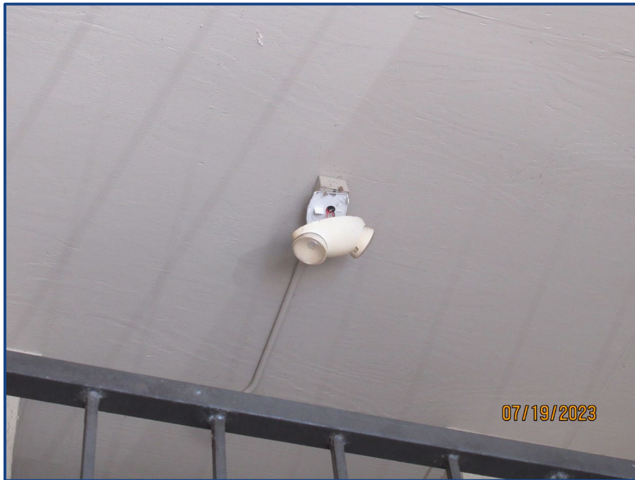
Photograph No. 22: Damaged emergency lighting fixture.
