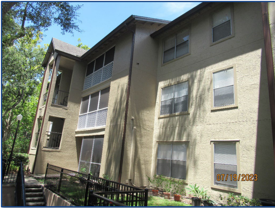
Photograph No. 11: View of the balconies and stairway on the southeast side of the building.
