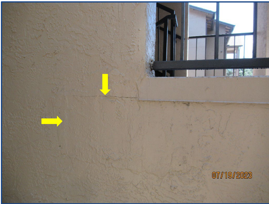
Photograph No. 12: Crack in the exterior wall stucco finish located on the southwest stairway.
