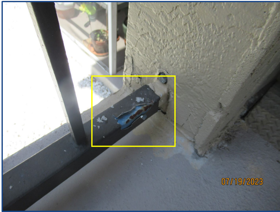
Photograph No. 19: Paint peeling and surface corrosion to the metal handrail located in the southeast stairway.
