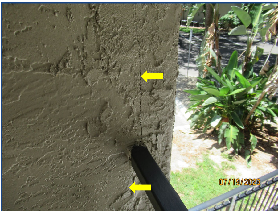
Photograph No. 14: Crack in the exterior wall stucco finish located in the southeast stairway.
