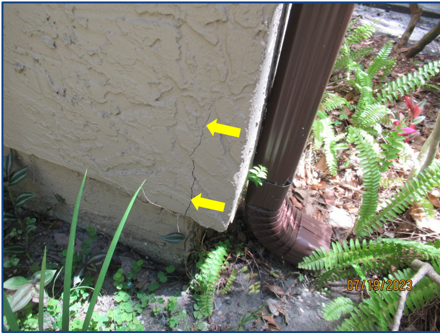
Photograph No. 13: Crack in the exterior wall stucco finish on the south side of the building.
