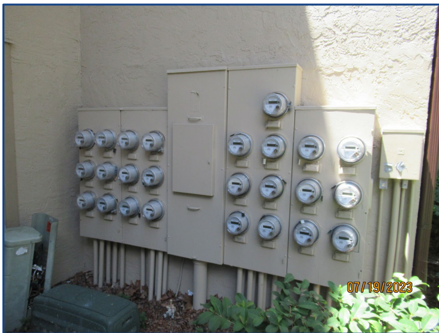
Photograph No. 20: Electrical panels.
