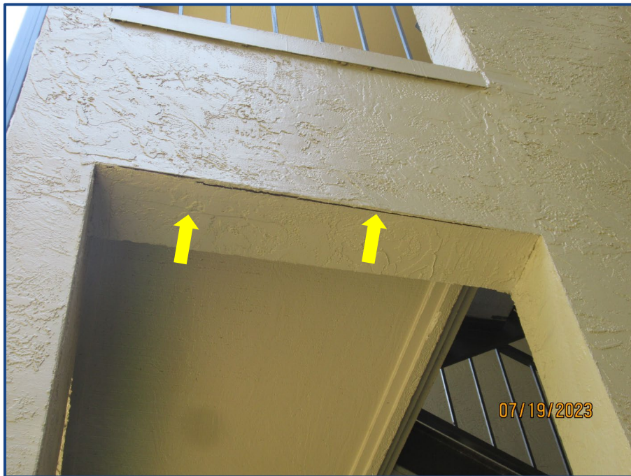
Photograph No. 16: Cracks in the exterior wall stucco finish located in the northeast stairway.
