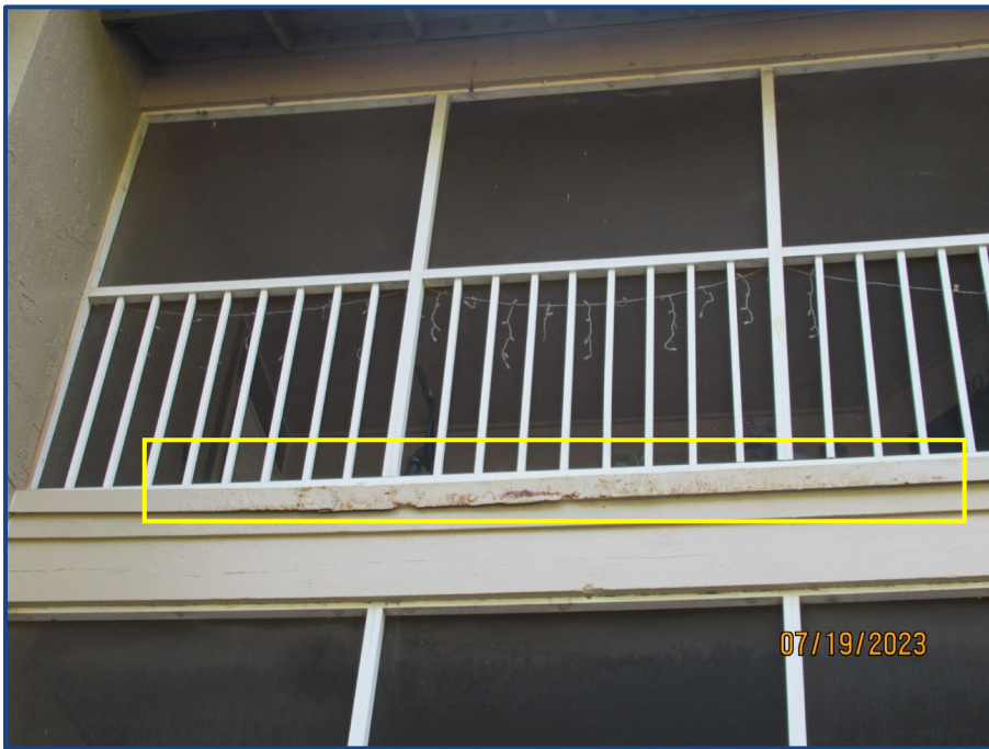
Photograph No. 10: Corrosion and separation of the metal flashing at the edge of the balcony slab on Unit 301.
