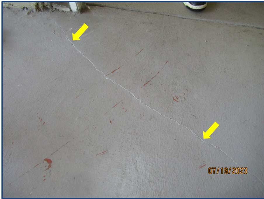
Photograph No. 16: Crack in the concrete balcony slab located on Unit 301.
