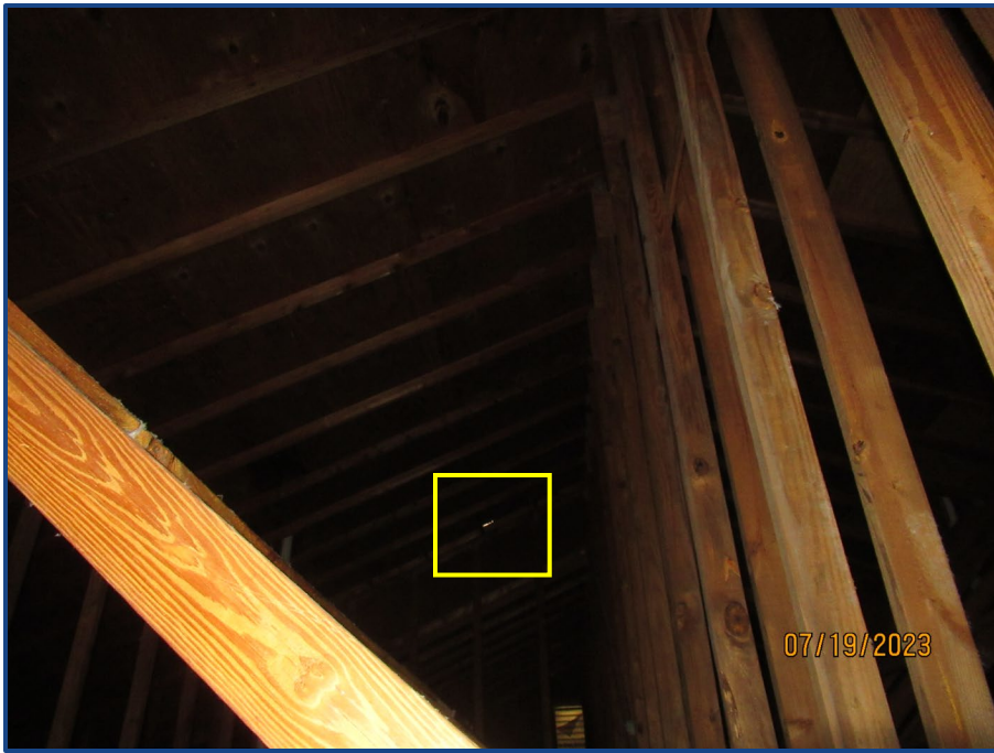
Photograph No. 7: A hole in the plywood roof sheathing.
