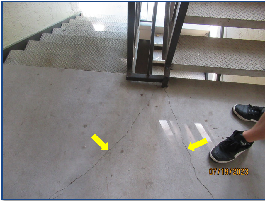
Photograph No. 15: Cracks in the concrete slab located on the 2nd floor.
