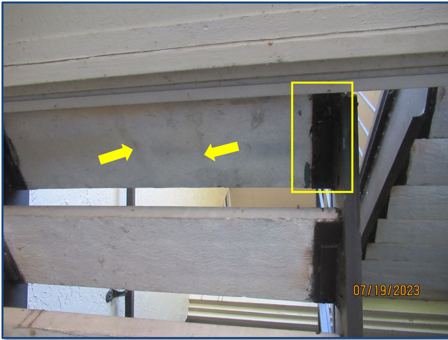
Photograph No. 19: Cracks in a concrete step and corrosion to the steel framing located in the west stairway.
