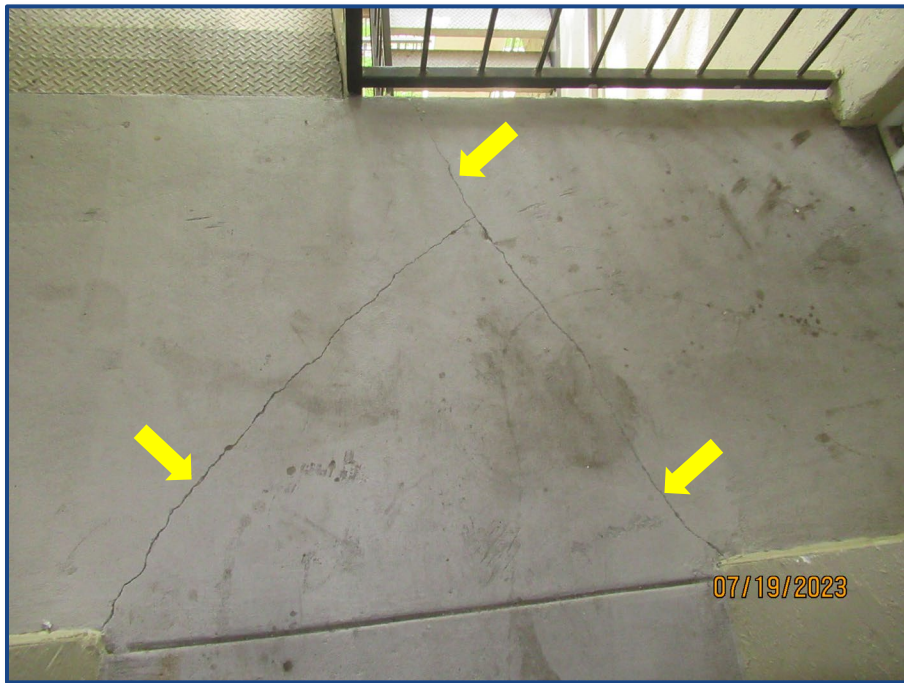
Photograph No. 14: Cracks in the concrete slab located on the 3rd floor.
