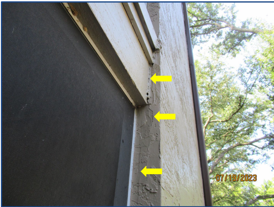
Photograph No. 12: Cracks in the exterior wall stucco finish located on the west side of the building.
