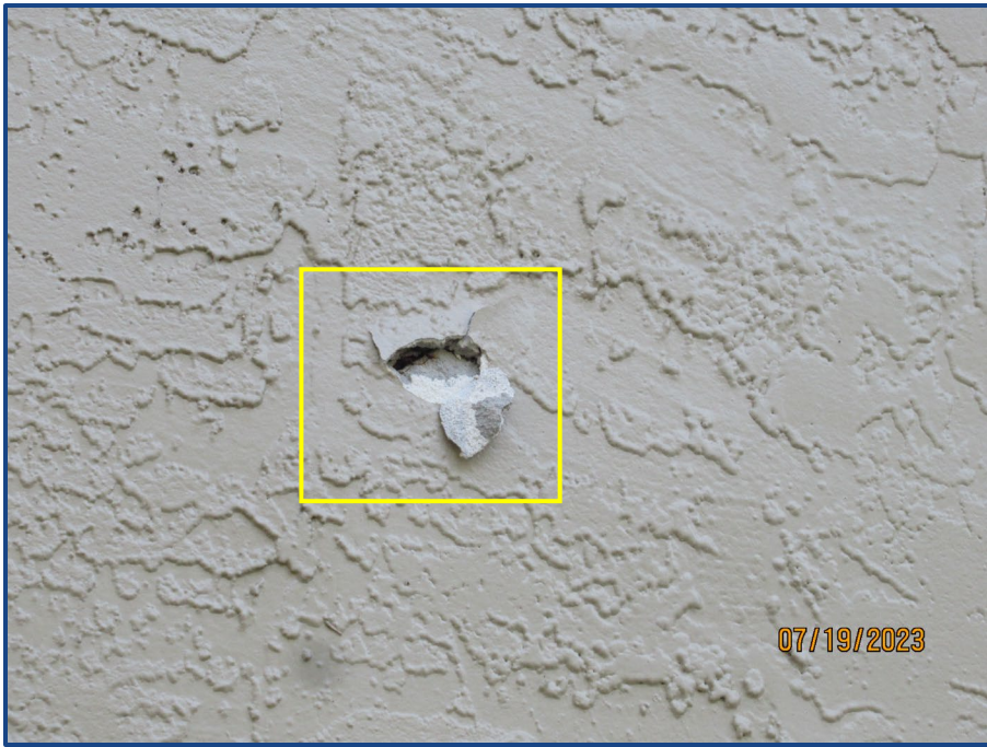
Photograph No. 11: Damage to the exterior wall stucco finish located above a window on Unit 102.
