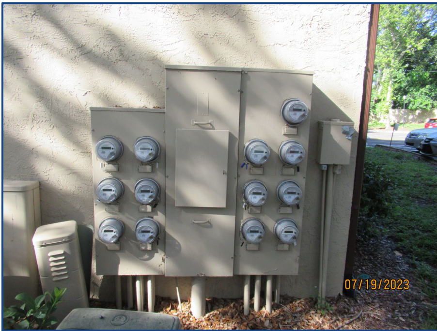
Photograph No. 20: Electrical meters.
