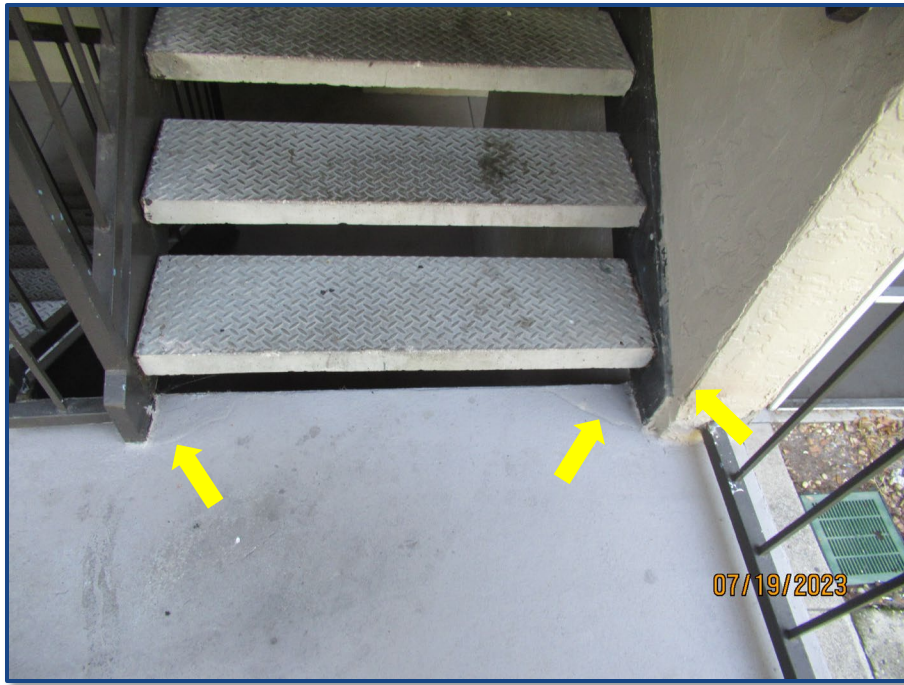
Photograph No. 13: Cracks in the exterior wall stucco finish and the stairway landing slab located in the west stairway.
