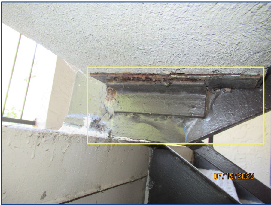
Photograph No. 18: Corrosion to the steel framing located in the west stairway.
