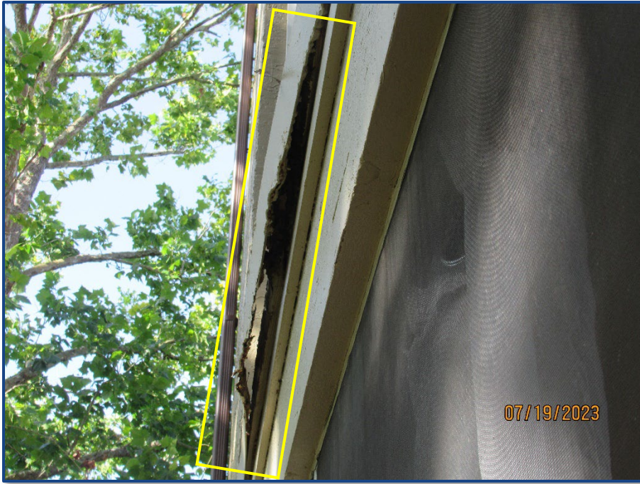
Photograph No. 9: Deterioration of the wood beam, corrosion, and separation of the metal flashing at the edge of the balcony slab on Unit 204.
