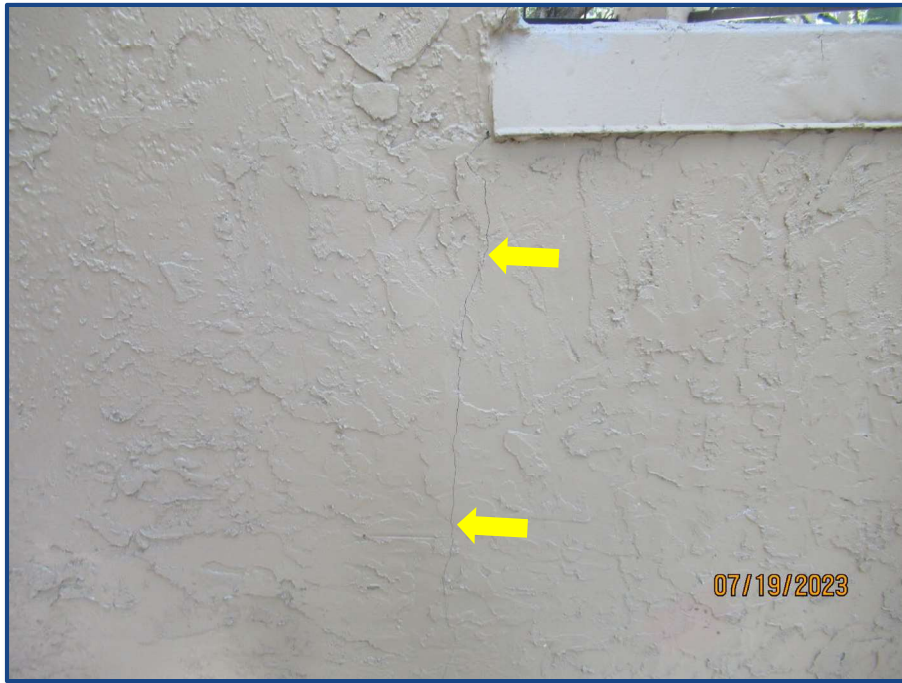
Photograph No. 17: Crack in the stucco wall finish located on the northeast stairway.
