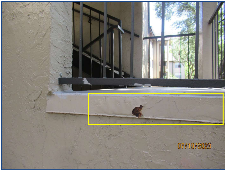
Photograph No. 12: Peeling paint and surface corrosion to the metal flashing at the edge of the northeast stairway landing slab.
