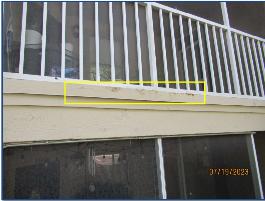
Photograph No. 13: Corrosion and separation of the metal flashing at the edge of the balcony slab on Unit 204.
