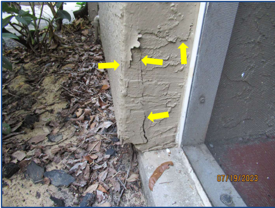
Photograph No. 15: Cracks in the exterior wall stucco finish and paint peeling at the exterior of Unit 106.
