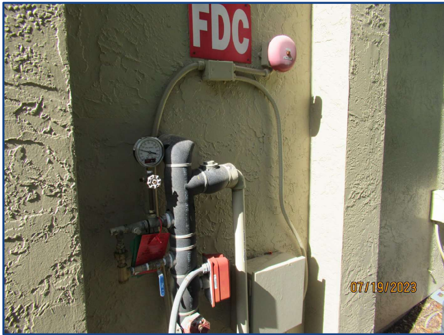
Photograph No. 26: Fire riser system and fire alarm.
