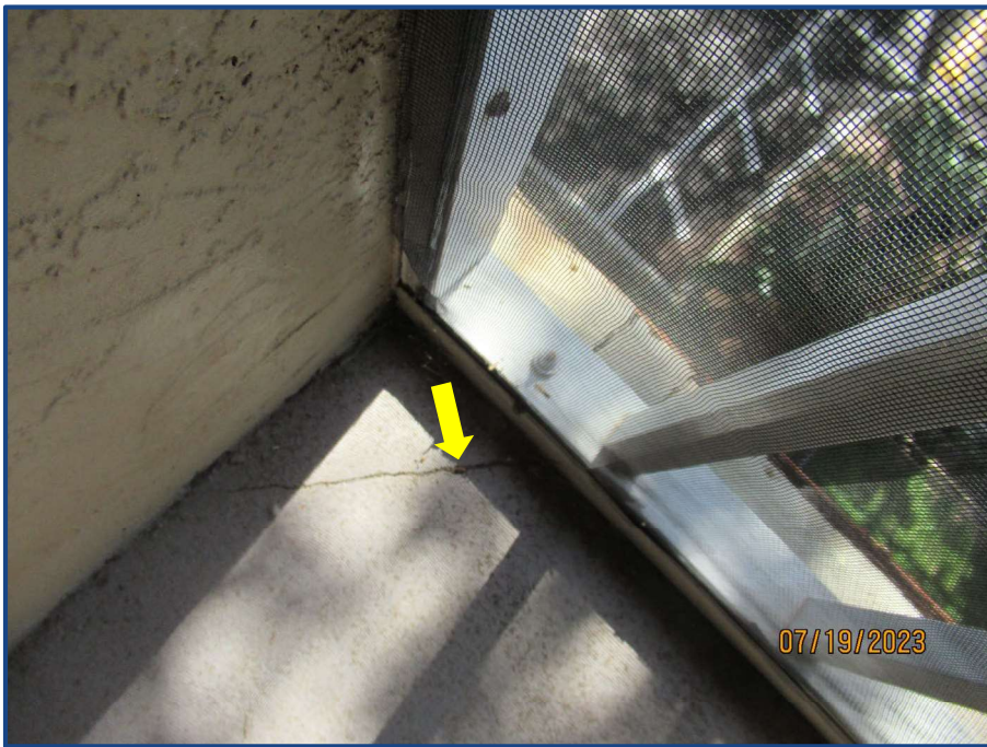
Photograph No. 22: Crack in the concrete slab located on the balcony of Unit 309.
