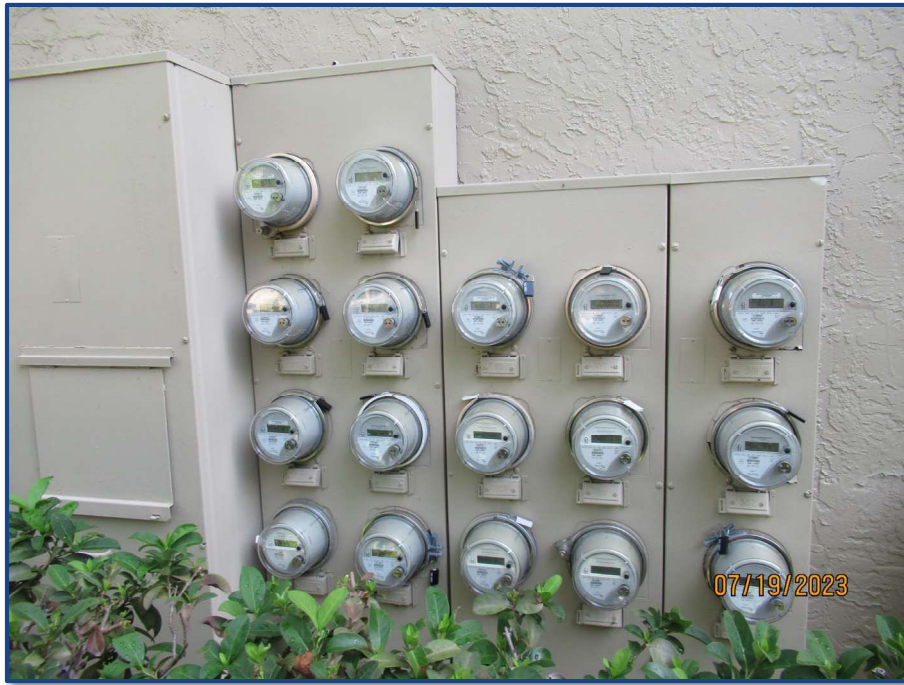
Photograph No. 25: Electrical meters.
