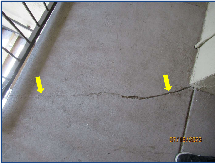
Photograph No. 21: Previously sealed crack in the concrete slab located at the north part of the building on the 3rd floor.
