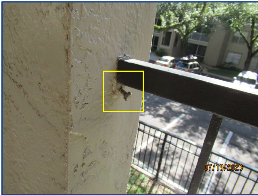
Photograph No. 24: A loose bolt located in the handrail connection in the northeast stairway.
