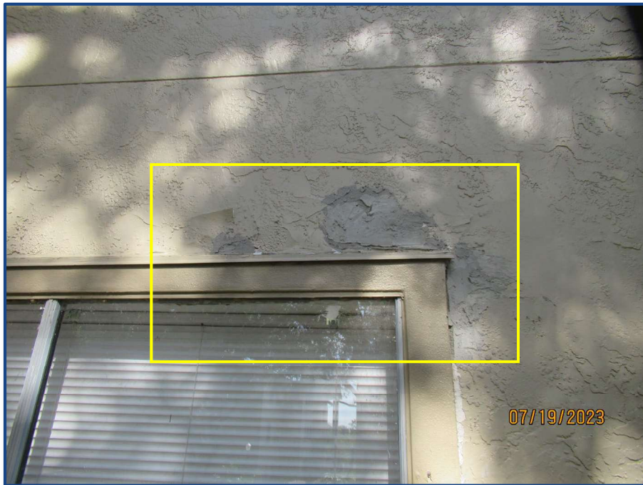
Photograph No. 18: Peeling of the paint finish and cracks in the exterior wall stucco patch located on the east side of the building.
