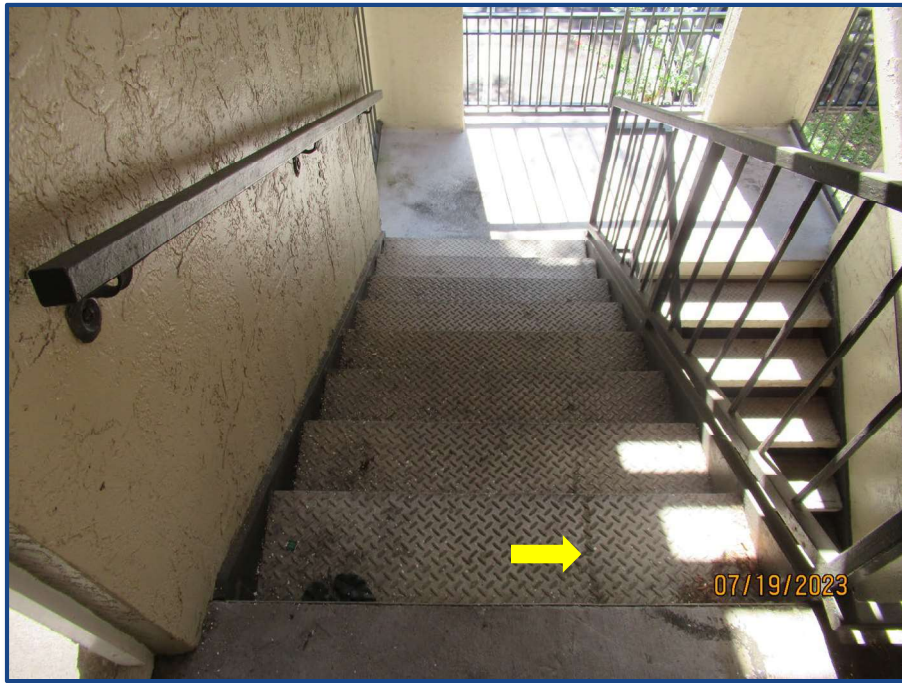
Photograph No. 23: Previously sealed crack in a concrete step located in the northeast stairway.
