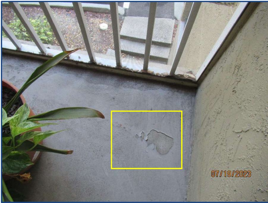
Photograph No. 19: Peeling of the balcony slab paint finish located on Unit 203.
