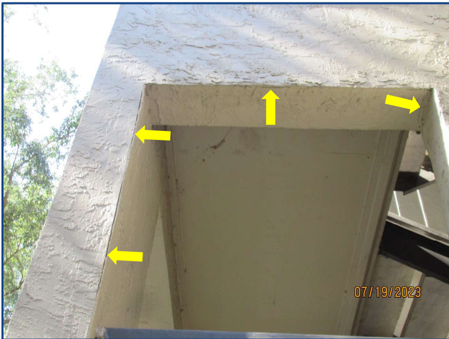
Photograph No. 16: Cracks in the stucco wall finishes located on the northeast stairway.
