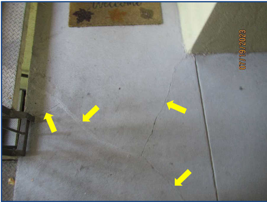
Photograph No. 20: Previously sealed crack in the concrete slab located at the north part of the building on the 2nd floor.
