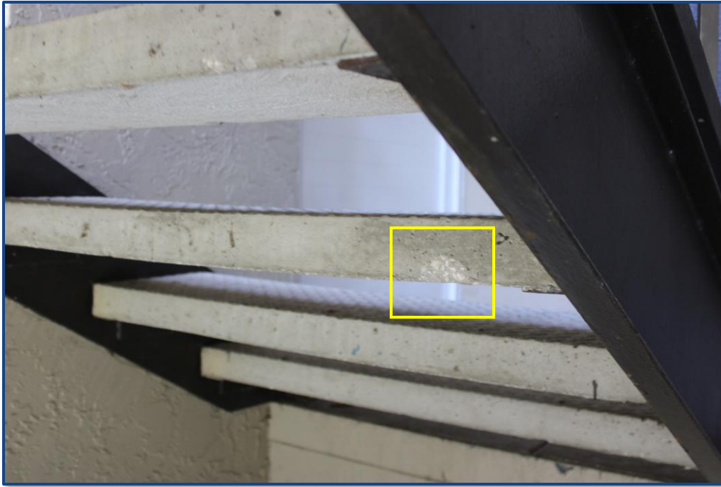
Photograph No. 11: Spalling in a concrete step located in the south stairway.
