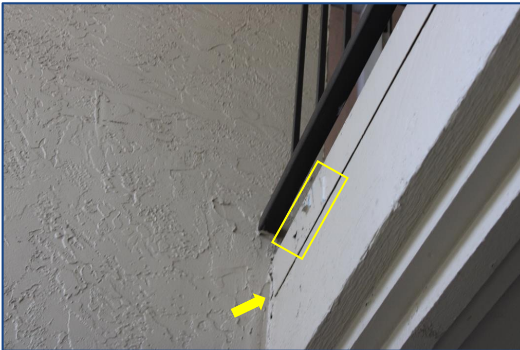
Photograph No. 6: Crack in the stucco wall finish and damage to the metal flashing at the edge of the stairway landing slab edge at the south stairway.
