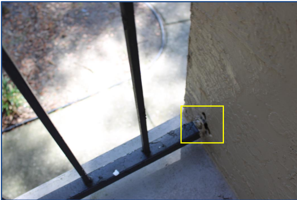
Photograph No. 12: Damage to the metal guardrail connection located in the south stairway.
