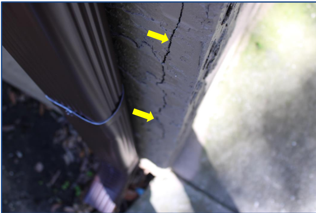
Photograph No. 8: Crack in the stucco wall finish located on the south stairway.
