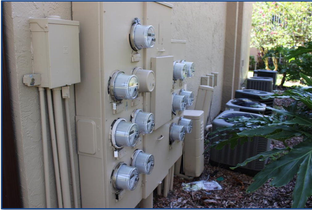
Photograph No. 13: Electrical meters.
