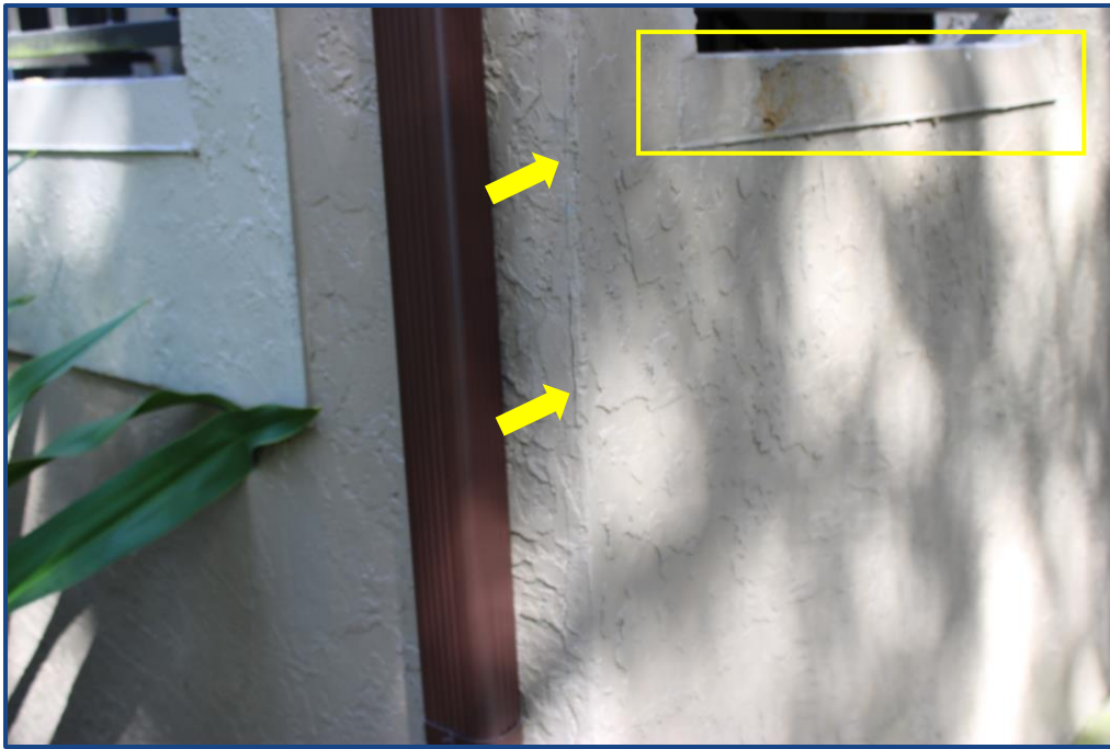
Photograph No. 7: Crack in the stucco wall finish and damage to the metal flashing at the edge of the stairway landing slab edge at the south stairway.
