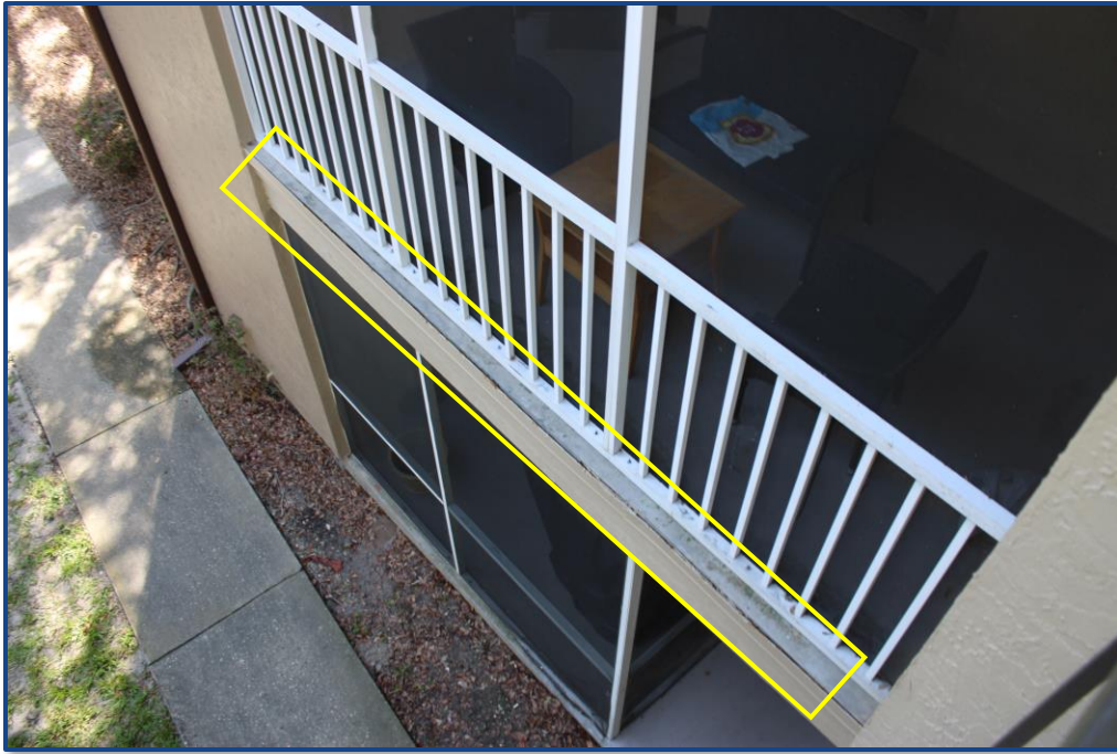
Photograph No. 5: Corrosion and separation of the metal flashing at the edge of the balcony slab on Unit 202.
