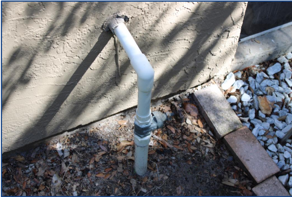
Photograph No. 14: Plumbing.
