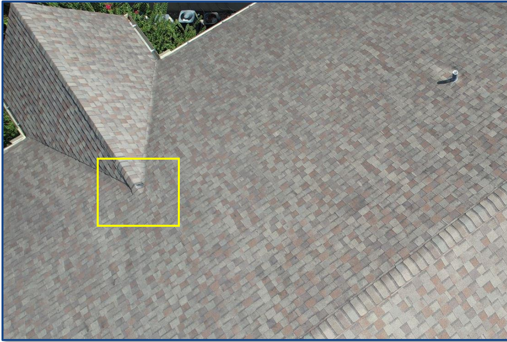
Photograph No. 3: View of damaged shingle at the north stairway gable ridge.
