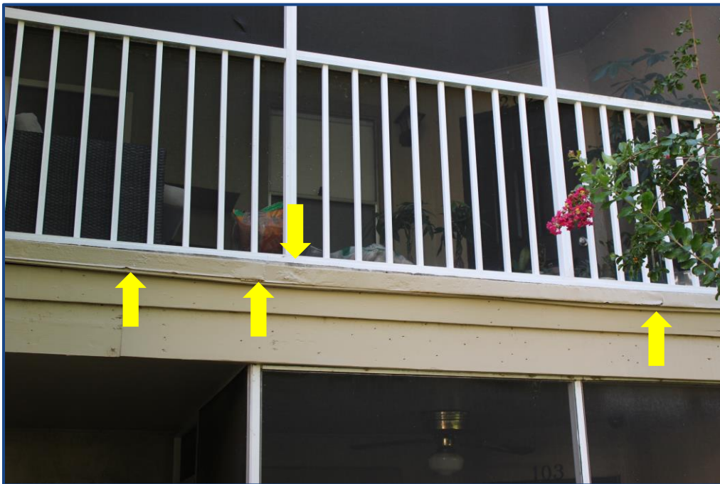
Photograph No. 16: Damage to the metal flashing located at the edge of the balcony slab on Unit 203.
