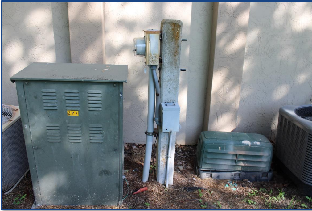
Photograph No. 19: Electrical boxes and meter.
