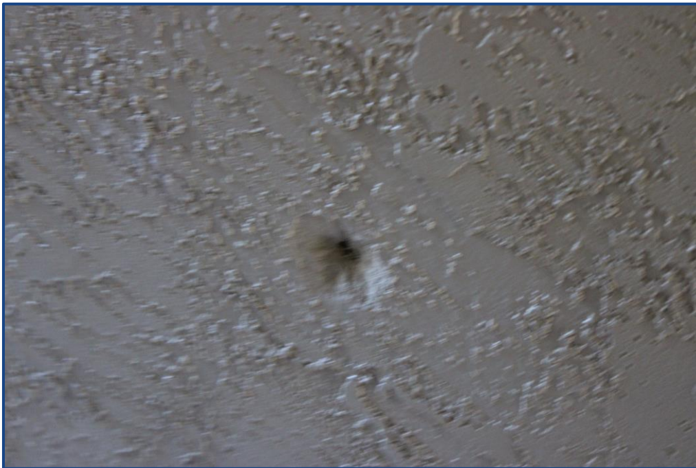
Photograph No. 8: View of damaged stucco in the exterior wall at the 2nd floor breezeway.
