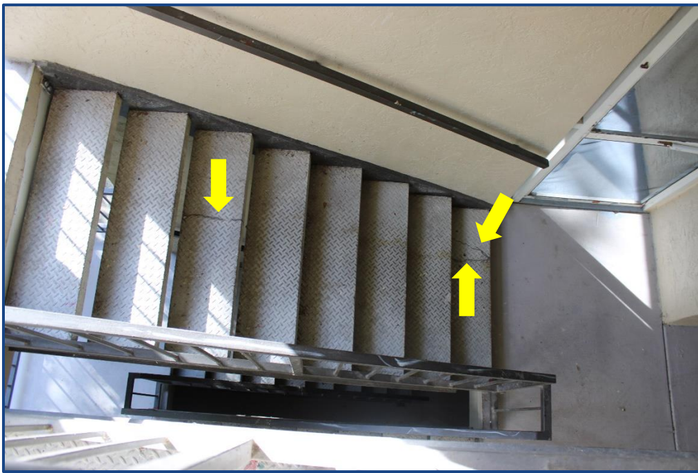
Photograph No. 12: Previously sealed cracks located in the concrete steps in the stairway.
