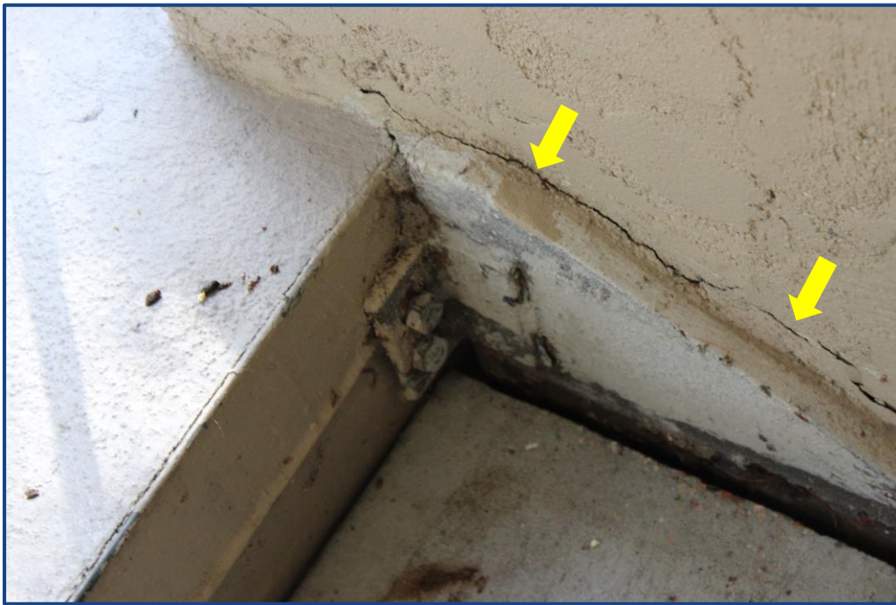
Photograph No. 14: View of cracks in the stucco finish located along the stairway riser.
