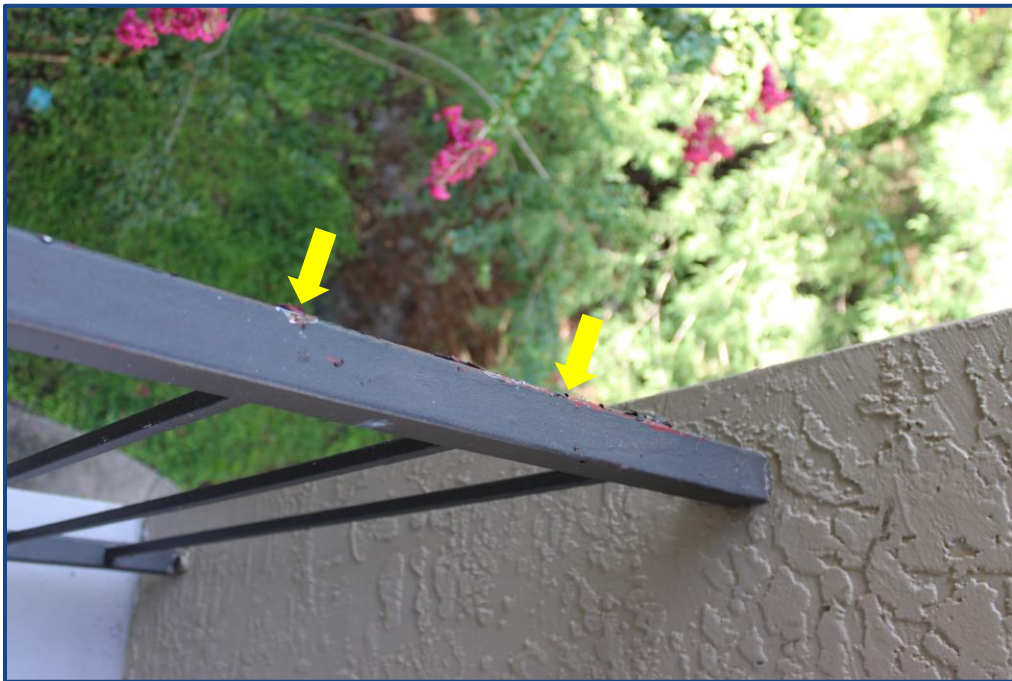
Photograph No. 10: Paint peeling located on the southwest stairway railing.
