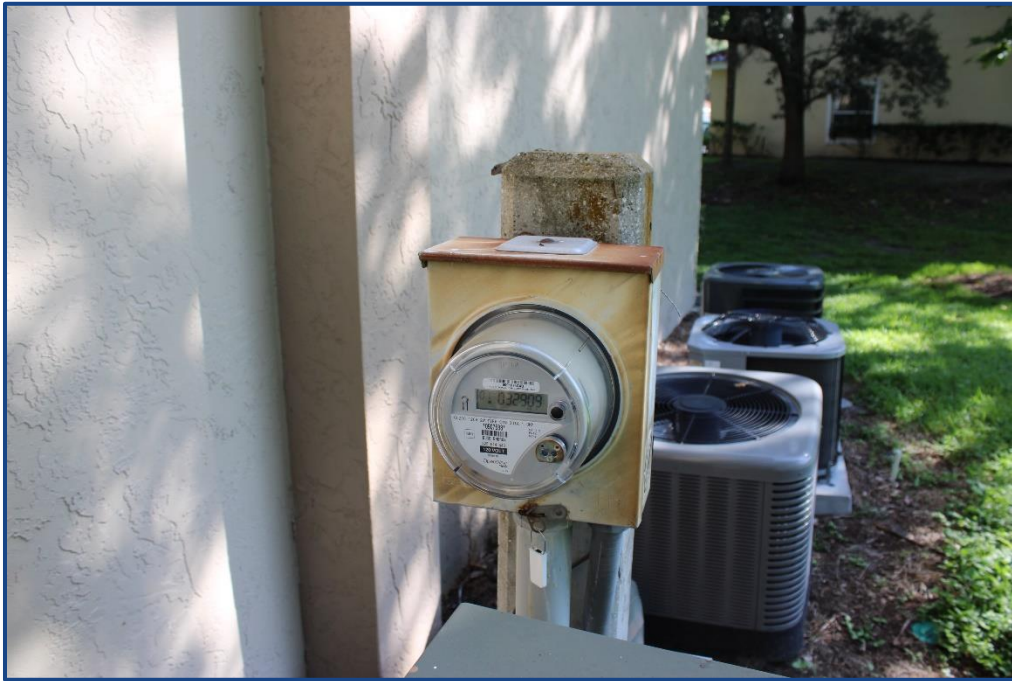
Photograph No. 20: Electrical meter.
