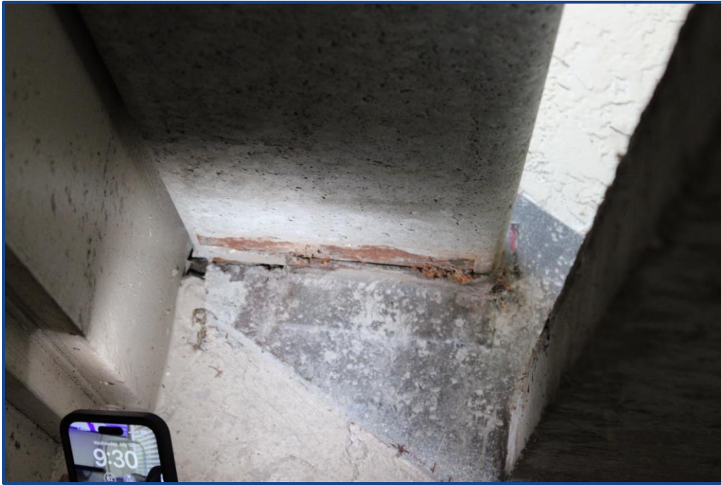
Photograph No. 15: Corrosion to the concrete step angle connection located in the stairway.
