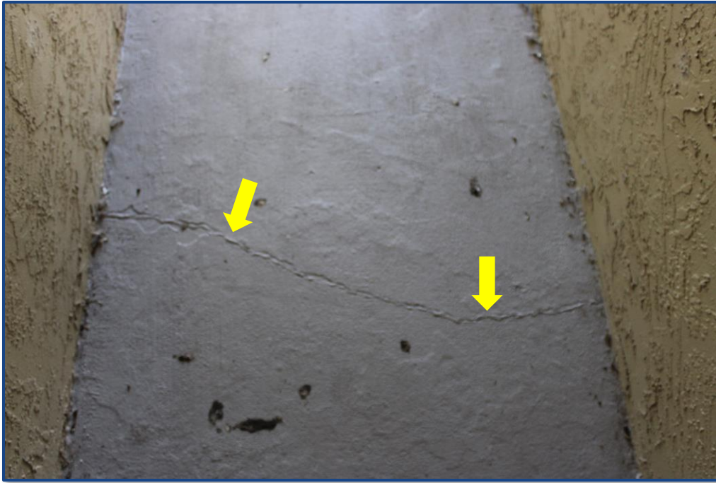
Photograph No. 11: Crack in the concrete slab located in the breezeway.
