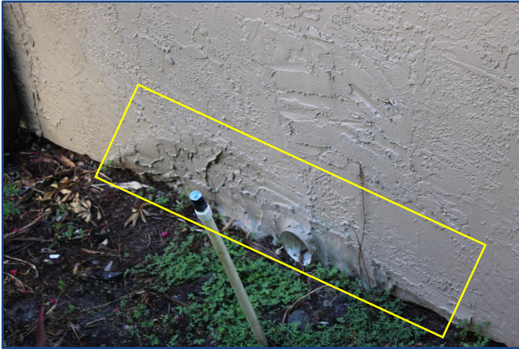
Photograph No. 17: Previously patched stucco around the scupper at the bottom of the stairway wall.
