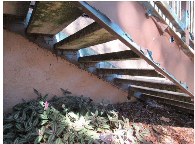
Finish deterioration and weathered stair treads and tread mounting angle
