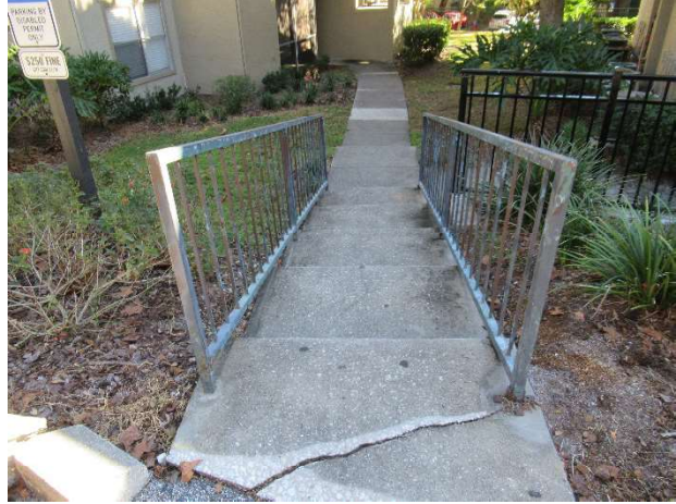
Deteriorated steel railings
