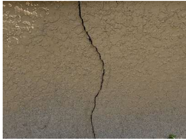
Perimeter wall crack
