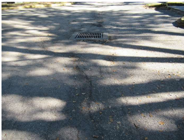
Centerline cracks and raveling
