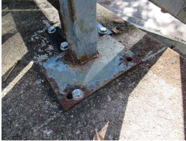
Rusted mount plate at staircase railings
