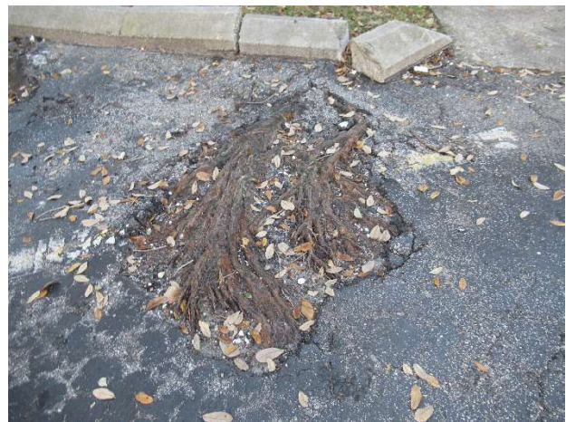
Completely deteriorated asphalt pavement
