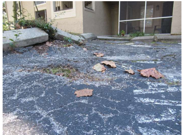
Severe settlement at parking areas
