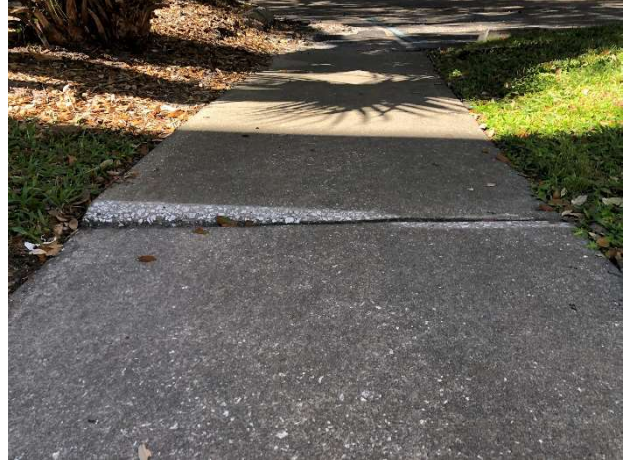
Trip hazard and previous repairs evident
