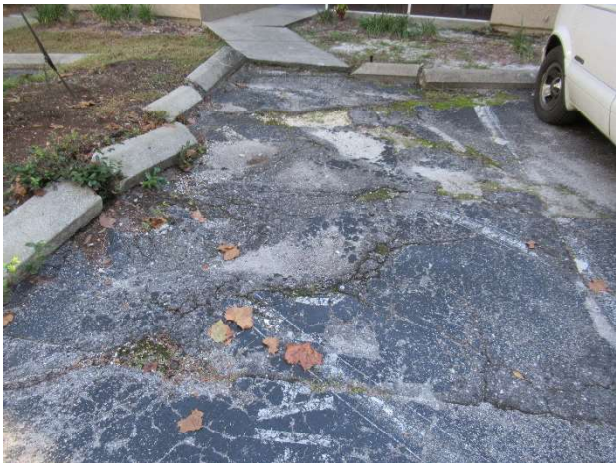
Severe settlement at parking areas
