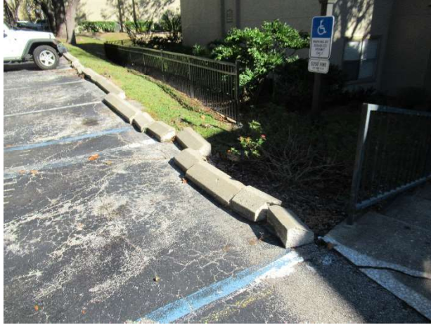
Broken and displaced curb
