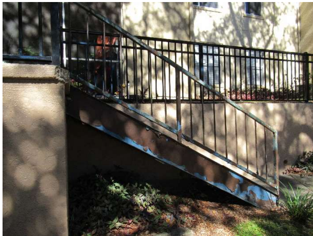
Deteriorated paint finishes at site staircases
