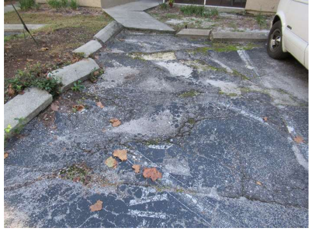
Broken and displaced curbs
