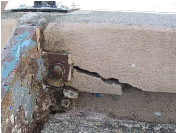
Deteriorated mount points and concrete cracks at the join of the site staircases and sidewalks
