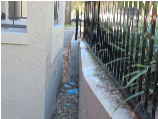
Retaining wall at this location has evidently been repaired since 2017
