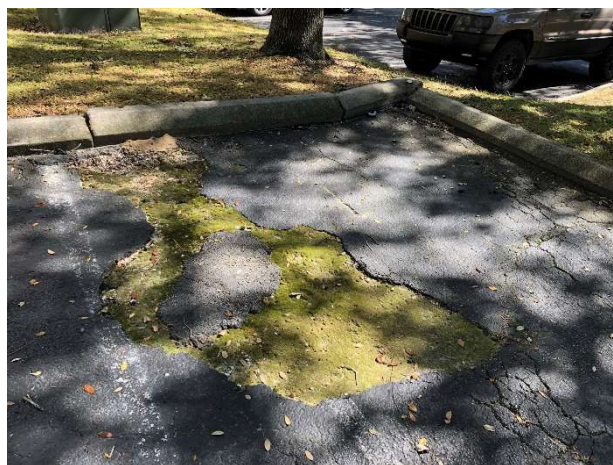
Pavement delamination and organic growth
