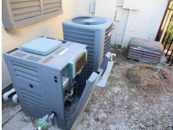
Spa heater missing cover
