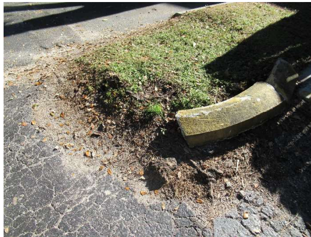
Broken and completed missing sections of curbs
