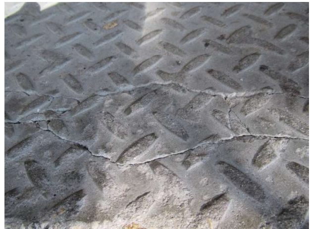
Severely cracked concrete treads
