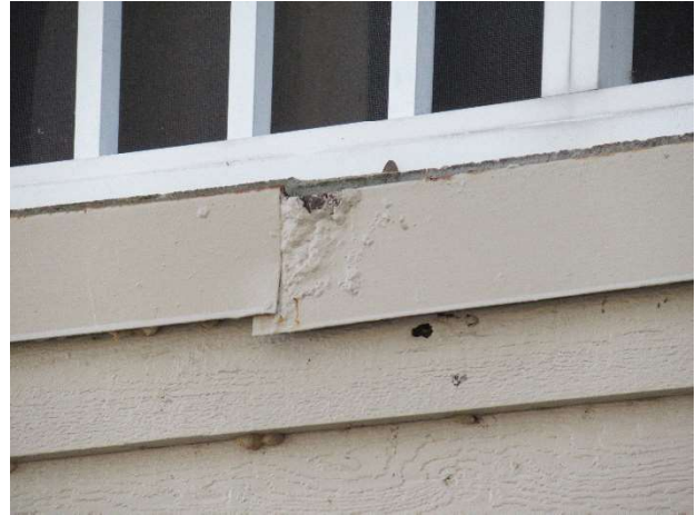
Misaligned and corroded flashing at balcony edge
