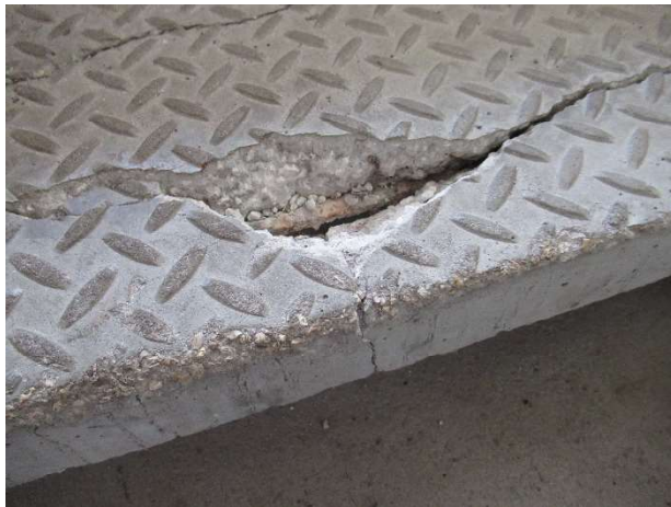
Exposed rebar at concrete treads
