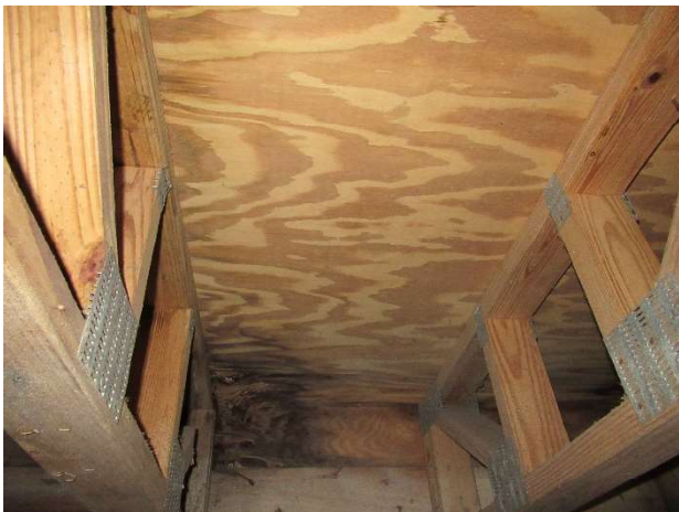
Wood rot at landing
