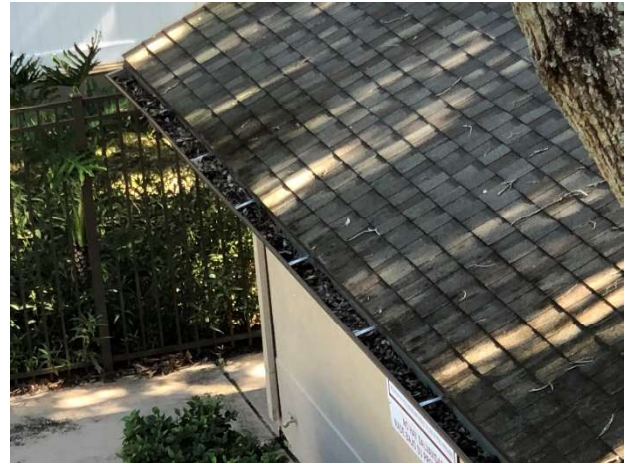
Debris accumulation at pool house gutters
