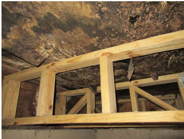
Severely rotted plywood at staircase landing (building 951)
