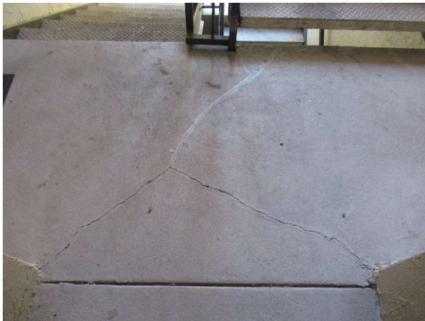
Cracks at breezeway
