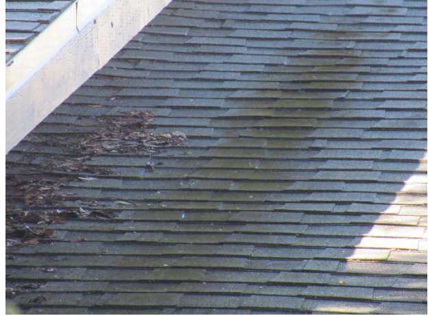
Debris accumulation and organic growth evident
