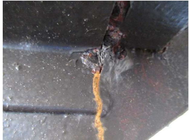
Isolated corrosion at tread mount angle
