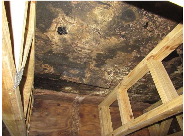
Severely rotted plywood at landing with evident replaced support frames
