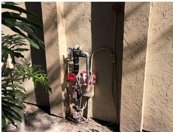
Fire suppression valves
