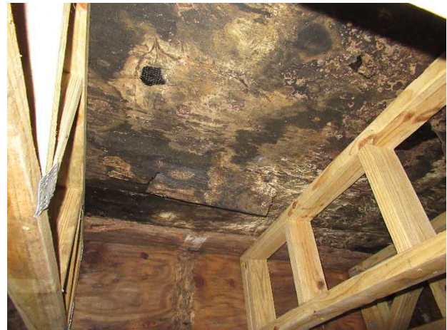
Severely rotted plywood at staircase landing (building 951)
