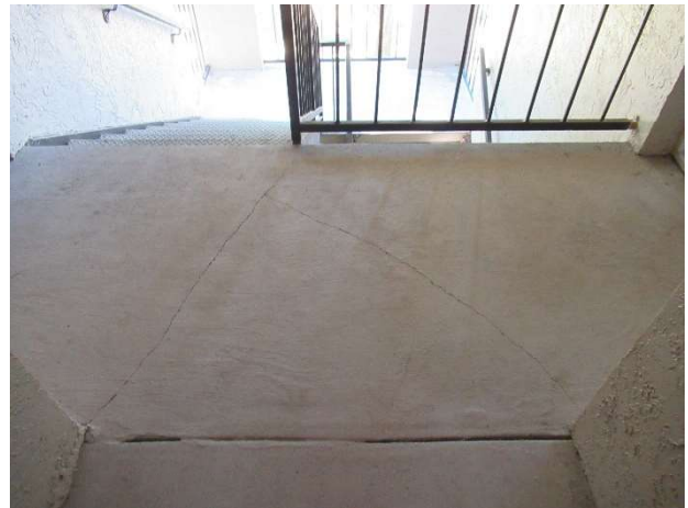
Cracks at breezeway
