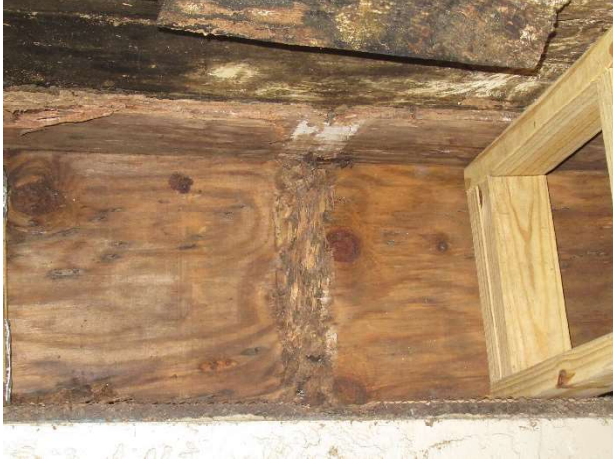
Wood rot at landing
