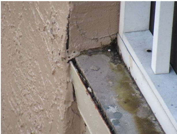
Detail view of balcony joint to building (note: stains)
