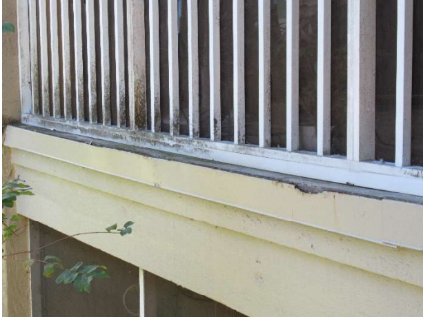
Damaged flashing and dirt accumulation at railings
