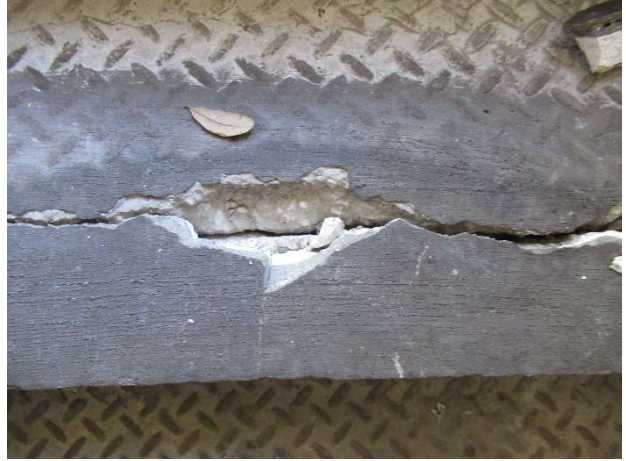
Severely cracked treads with previous repairs evident
