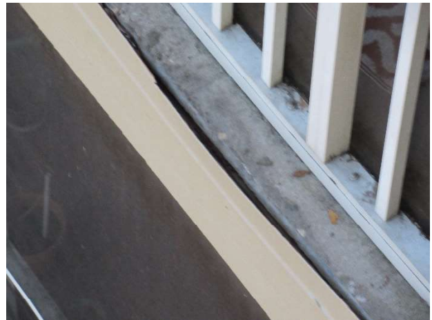
Misaligned flashing at balcony edge
