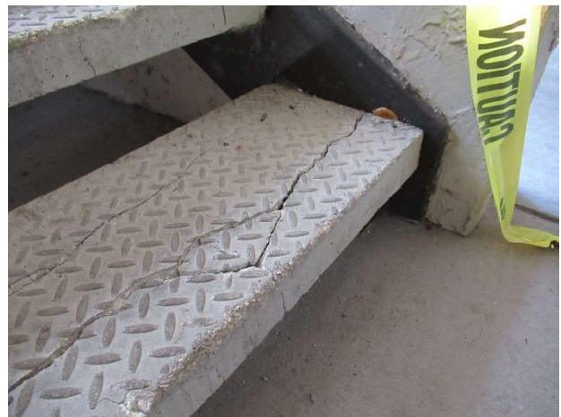
Severely cracked concrete treads
