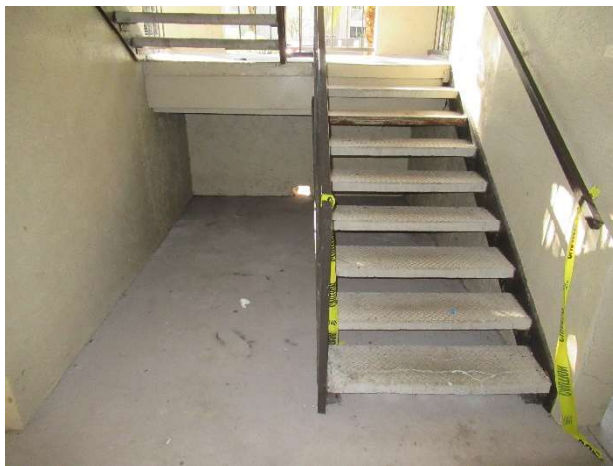
Staircase with torn safety tape
