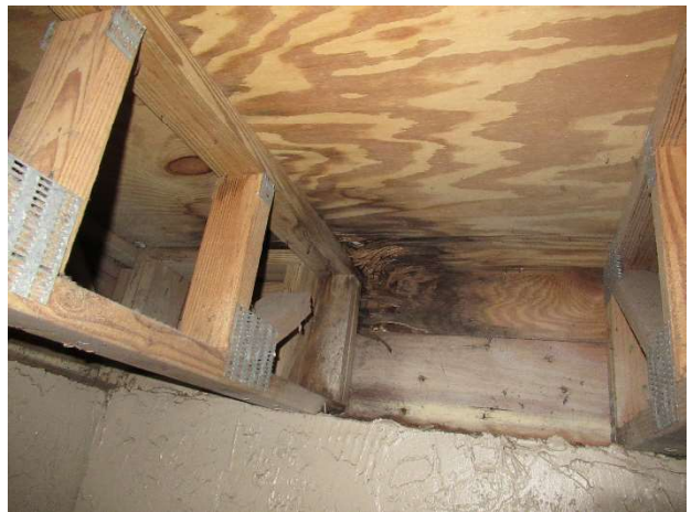
Wood rot at landing
